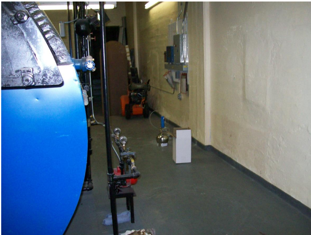
PHOTO 19: Northward view of sub-slab sample C-SS-1 in CESCO boiler room.
