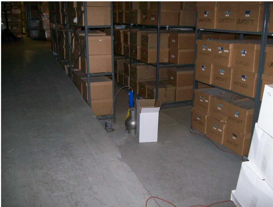
PHOTO 21: Northward view of sub-slab sample C-SS-3 in northern portion of CESCO basement.
