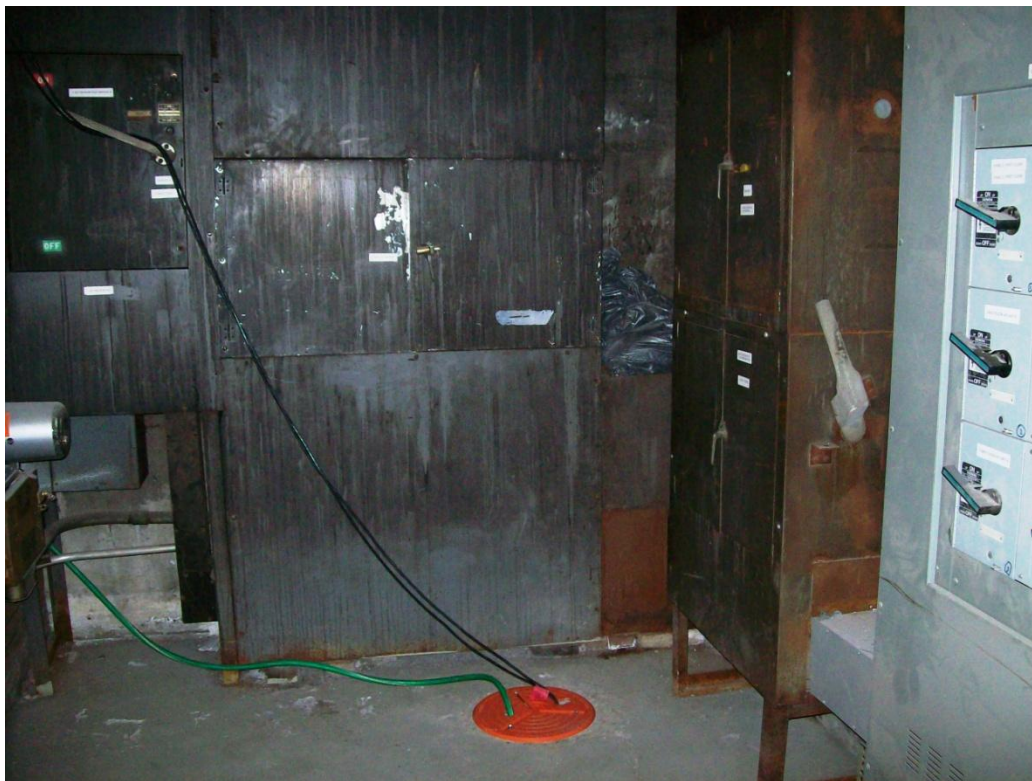
PHOTO 26: Westward view of electrical room in Bark Frameworks basement .
