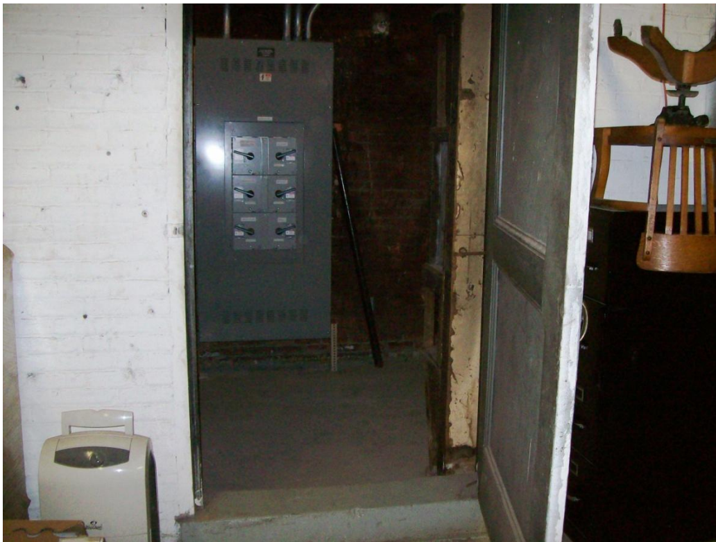
PHOTO 25: Northward view of electrical room in Bark Frameworks basement.
