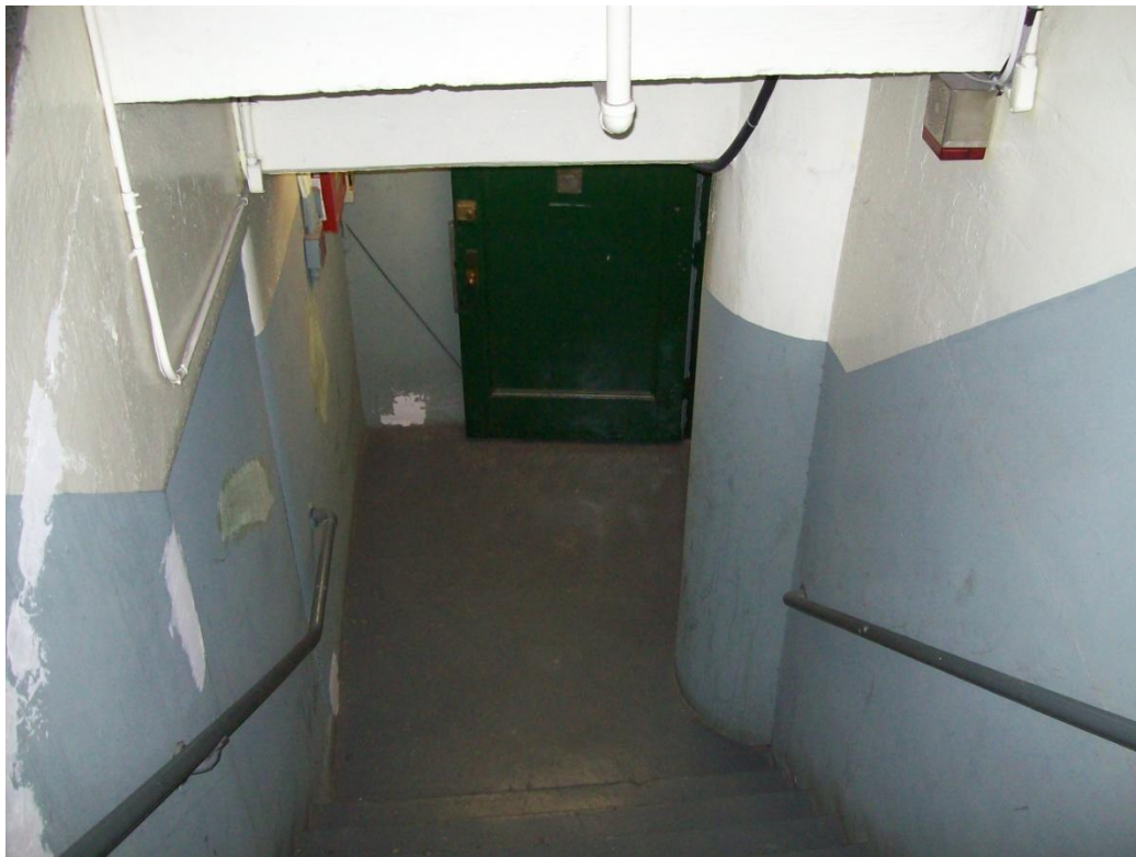
PHOTO 7: Northward view of stairway and entrance to CESCO Building basement from 44 th Road .
