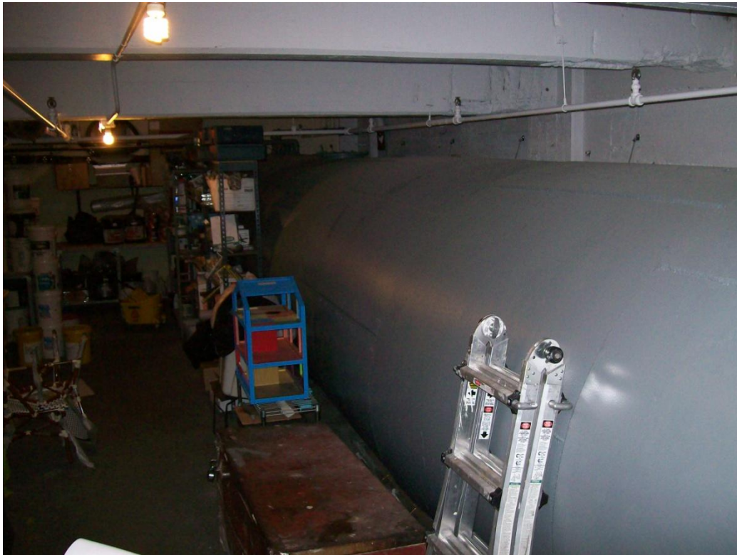
PHOTO 10: Eastward view of 10,000 gallon oil tank and paint/primer storage from maintenance office.
