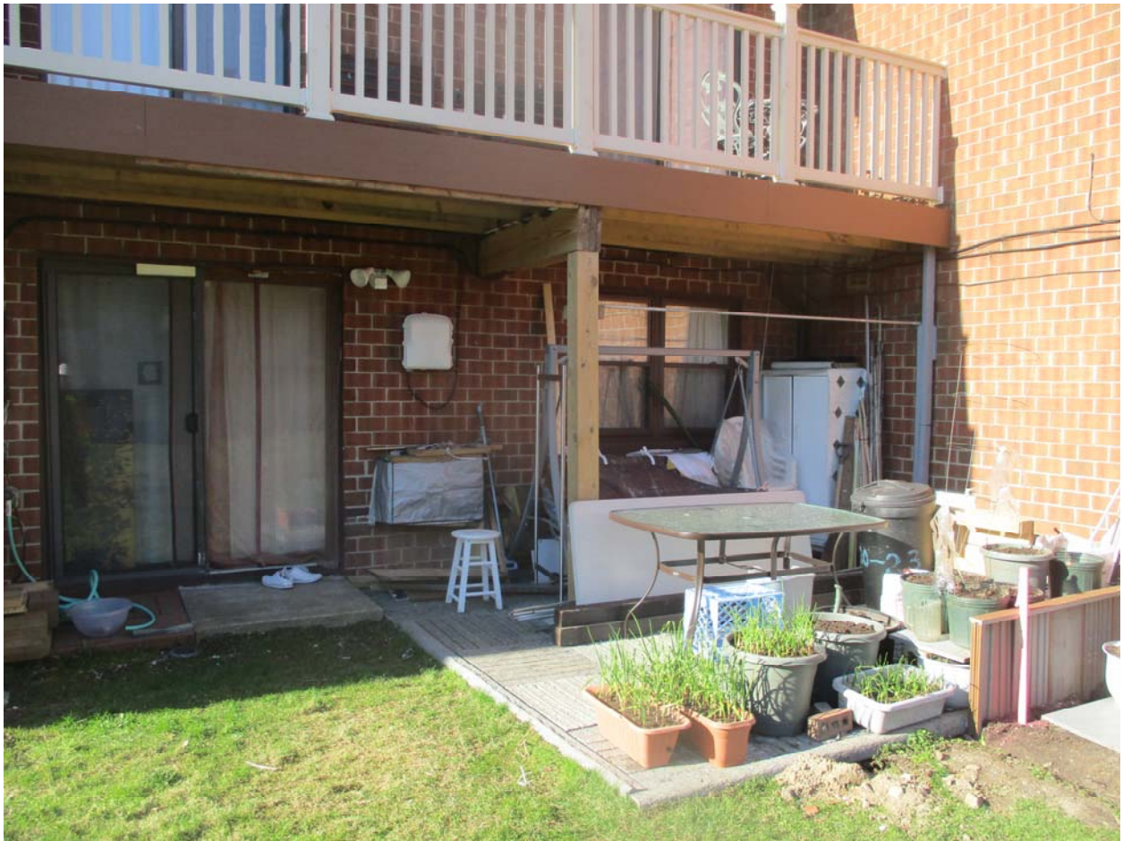
Yard 18: All hard surfaces in this Yard shall be protected, with the exception of the red brick patio to the left of the poured concrete patio.
