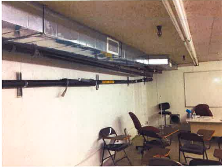
Photos 1-2 (October 12, 2018): View of installed piping (cast iron) within cellar.
