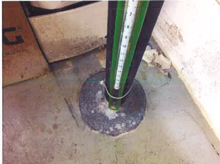
Photo 5 (October 12, 2018): View of suction pit/point through grade slab.
