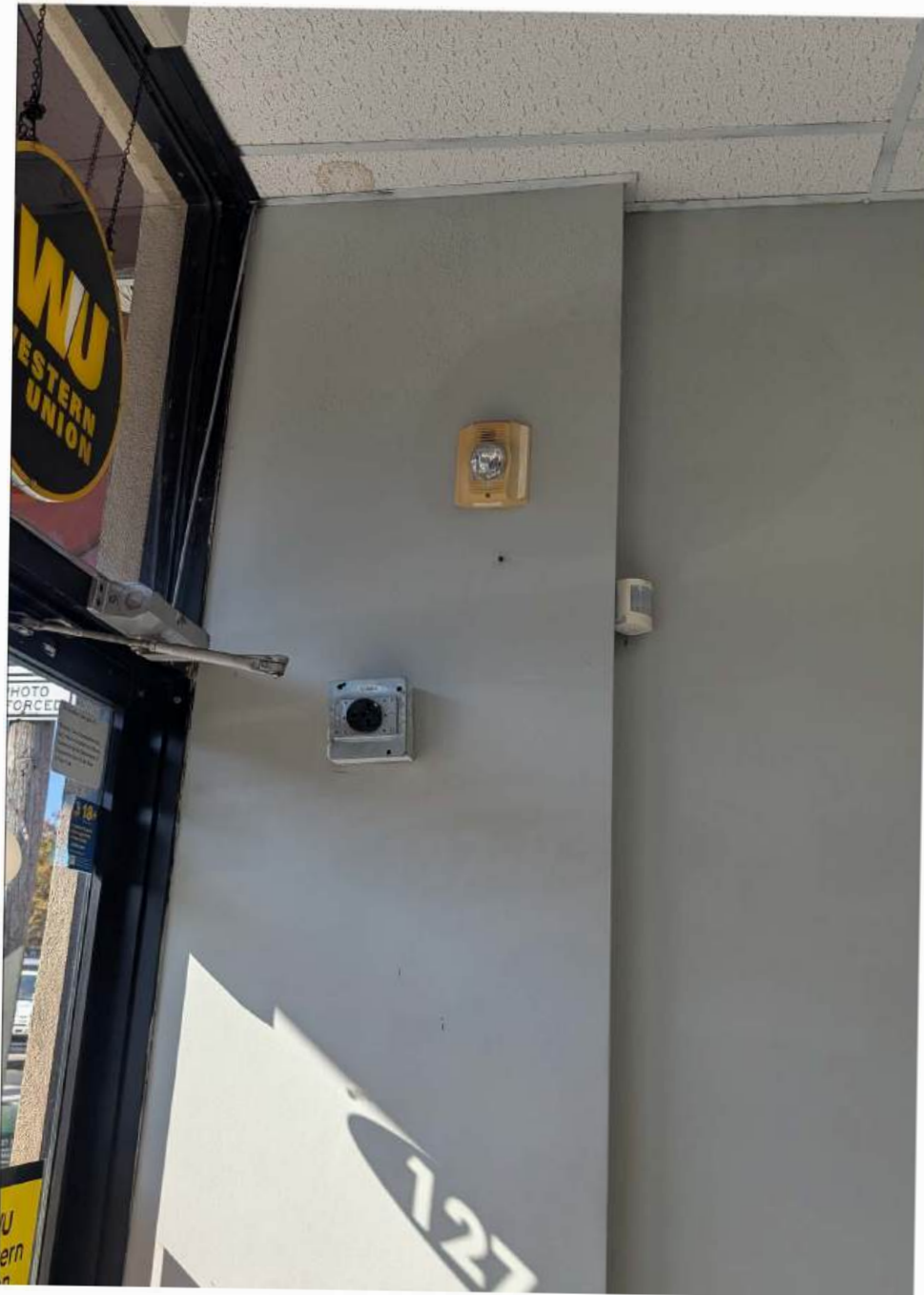
SSDS WARNING LIGHT AND ALARM IN UNIT 127-03
