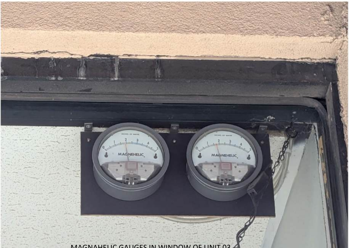
MAGNEHELIC GAUGES IN WINDOW OF UNIT 03
