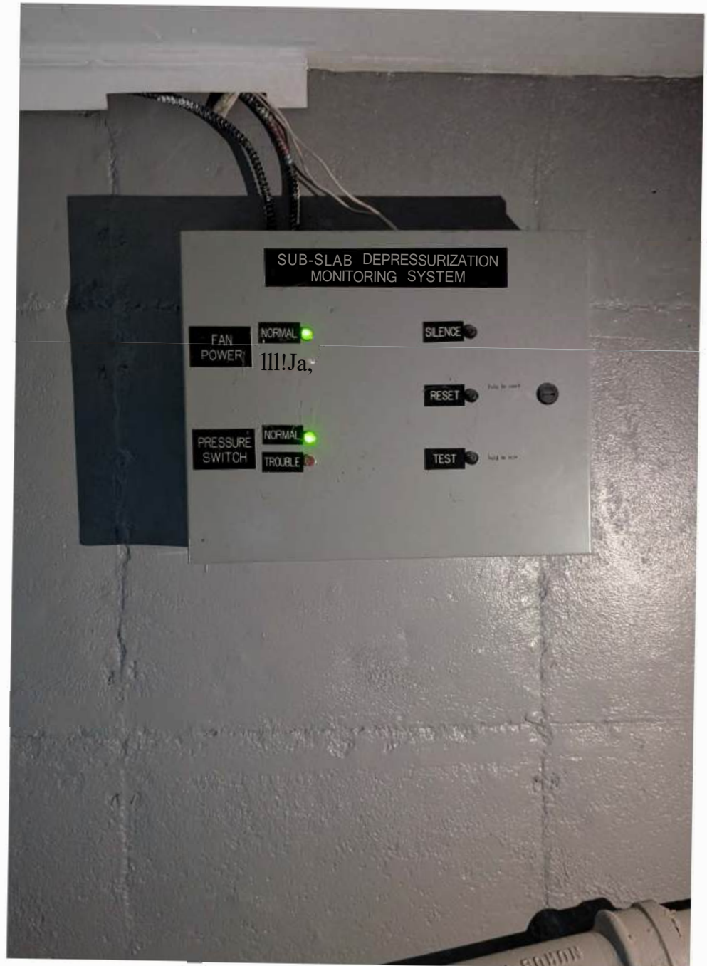
SSDS CONTROL PANEL IN BASEMENT OF UNIT 127-03
