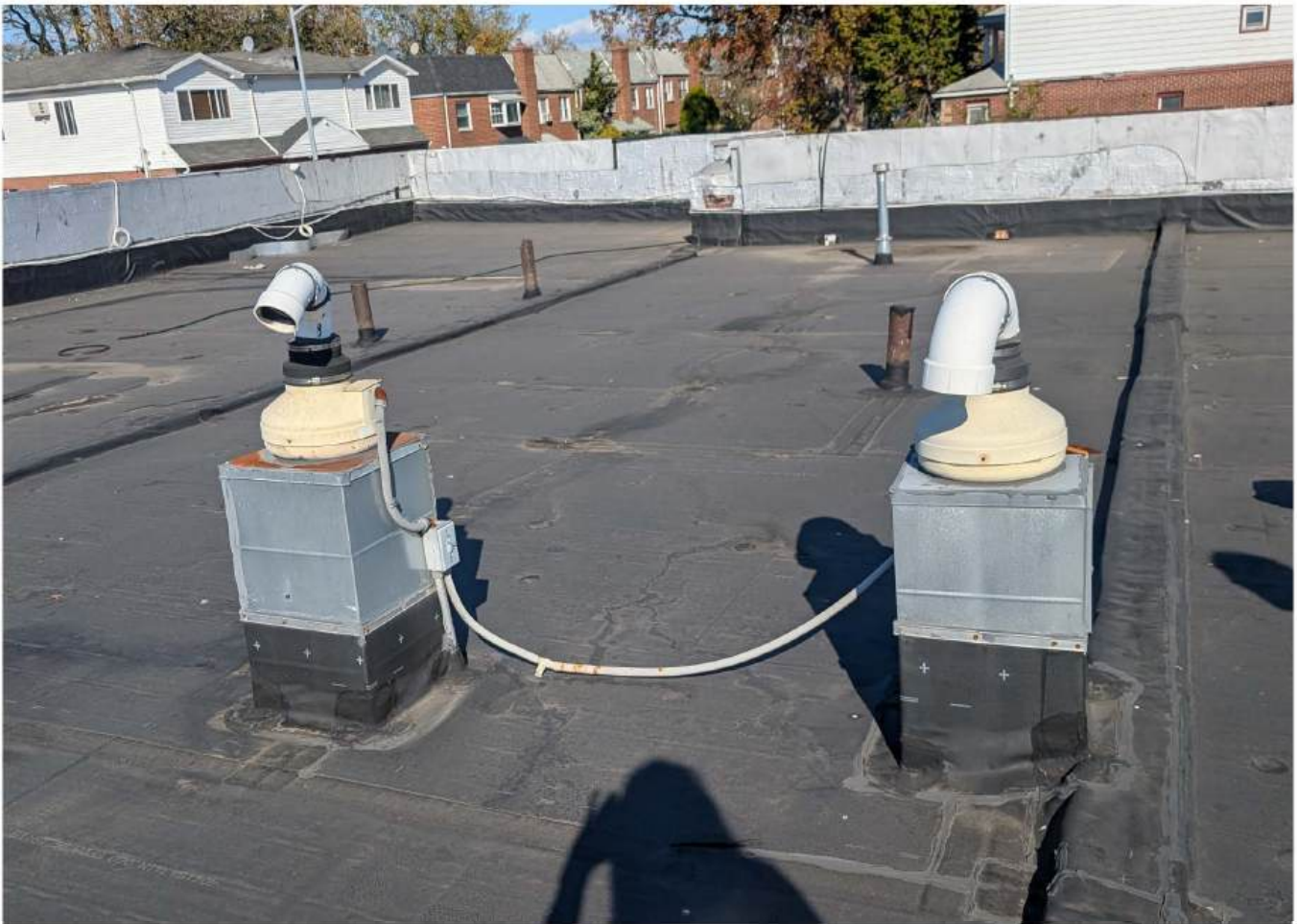
SSDS FANS ON ROOF
