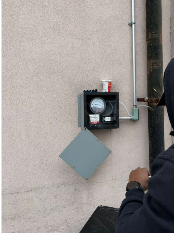
Dwyer magnehelic gauge and alarm at SVE system
