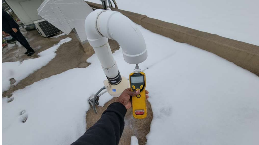
Organic vapor measurement at the effluent from SSDS Pit 1 to SSDS Pit 3
