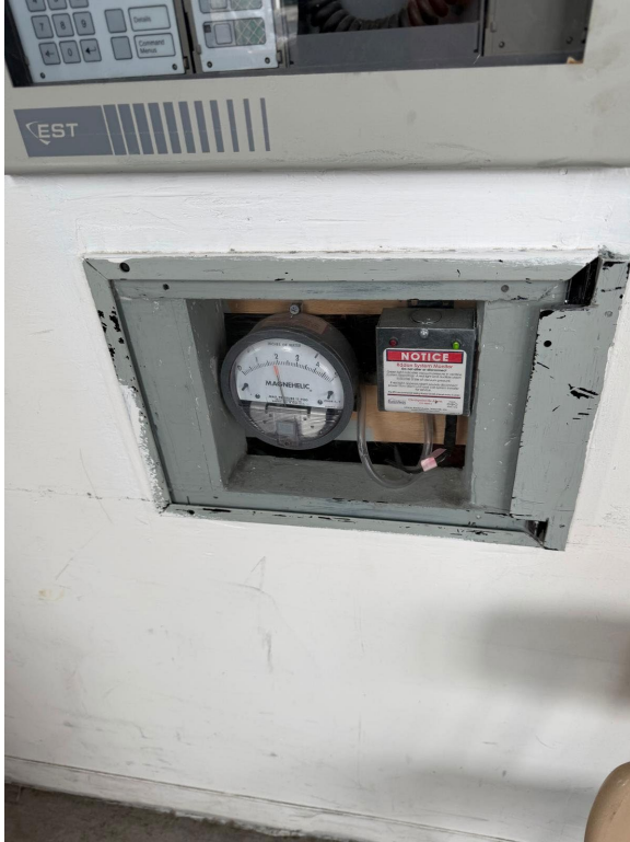
Dwyer magnehelic gauge and alarm at SSDS Pit 4
