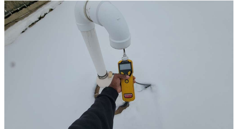
Organic vapor measurement at the effluent from SSDS Pit 4
