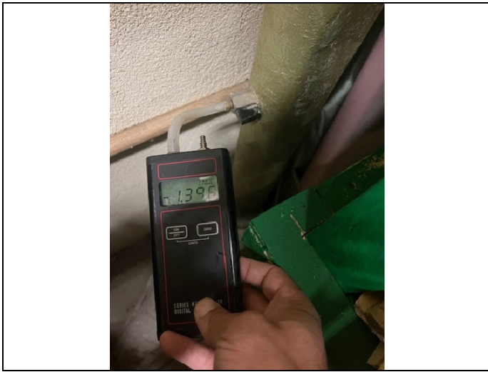
7. Measuring Pressure in fan P-1
