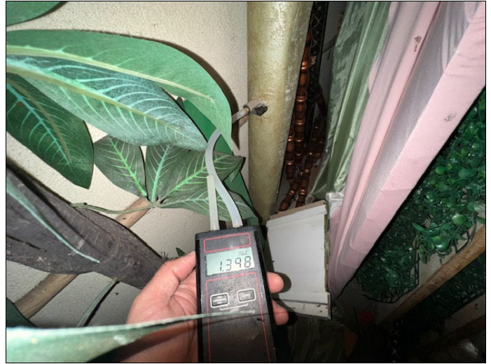
2. Reading from SSD Riser Pipes
