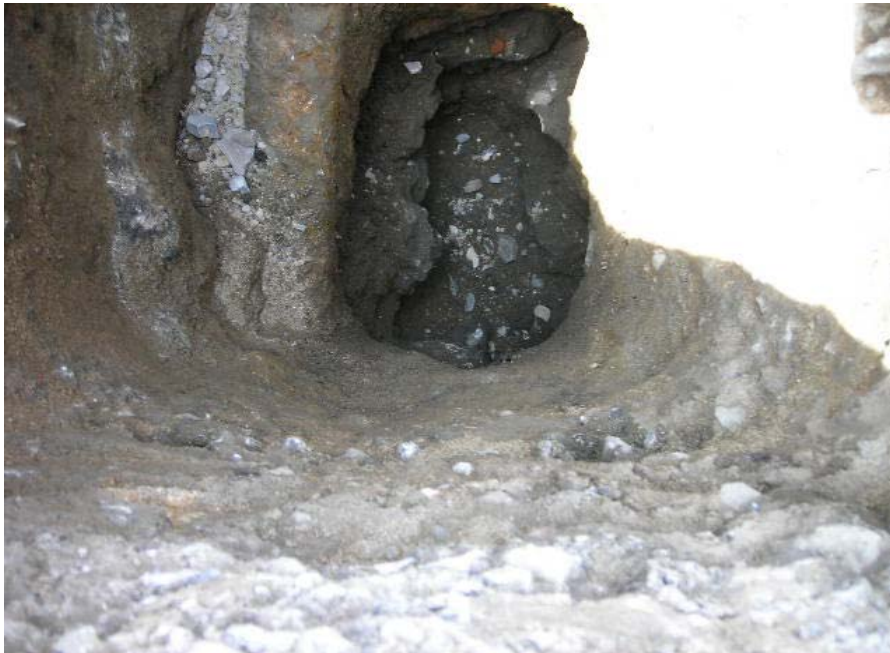
Above: Hollow concrete encountered at 4 ft bgs.
