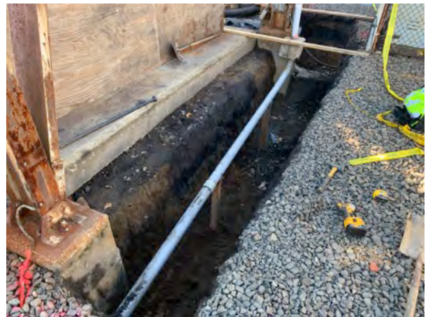
All exposed conduit is supported with wood.
