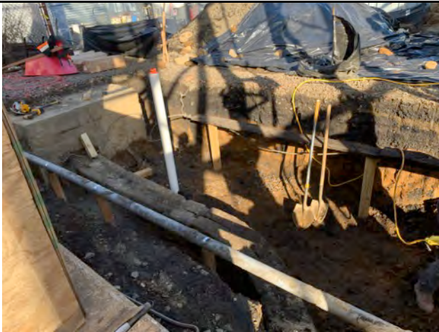
Wooden supports for conduit.
