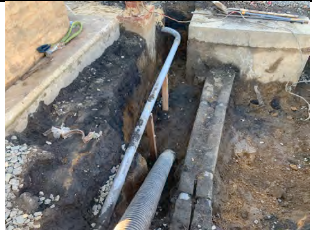
Aarco supporting all uncovered conduits.
