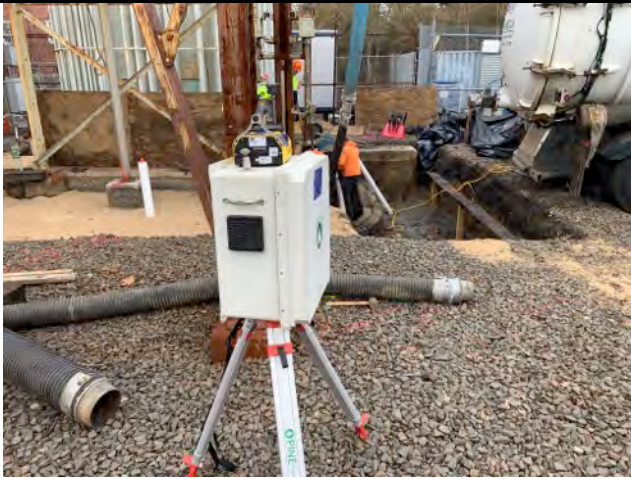
View of work zone camp monitor.
