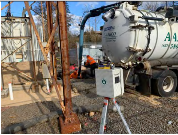
View of work zone camp monitor.
