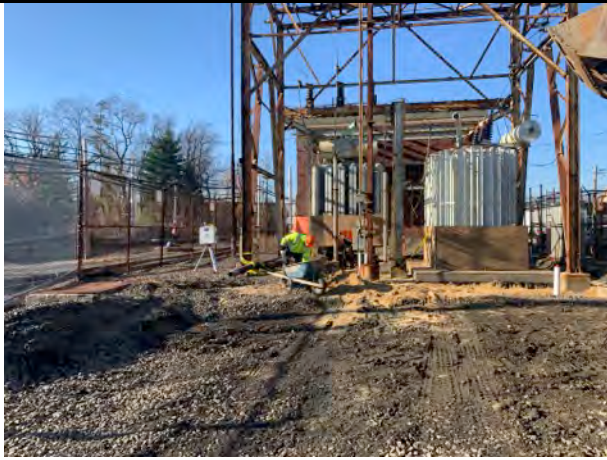
View of work zone camp monitor.
