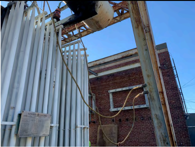
LIRR Substations grounding wire installed on transformers.
