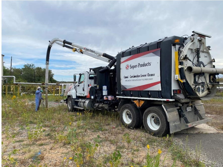
Photo 1: View of Entact hydro-vac truck pot holing utilities in IRM 1 Eastern Area, Excavation 5, facing southeast.
