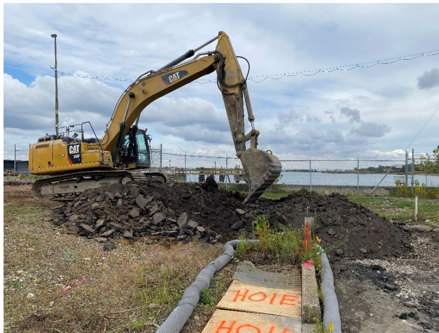
Photo 2: View of Entact operator stockpiling asphalt in IRM 1 Eastern Area, Excavation 4 zone, facing north.
