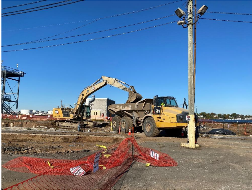
Photo 1: View of rock truck being loaded with soil to be stockpiled and prepped for disposal, in IRM 1 Western Area, Excavation 1, facing west
