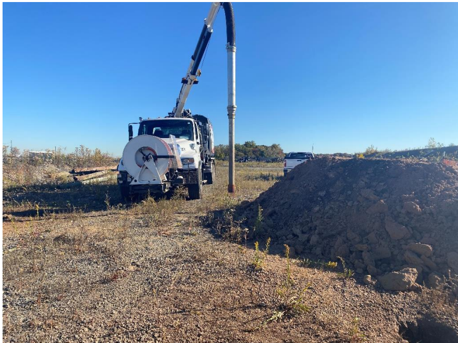
Photo 2: View of pot holing activities using the Hydro-Vac Truck in Excavation 9, IRM 1 Central Area, facing north.
