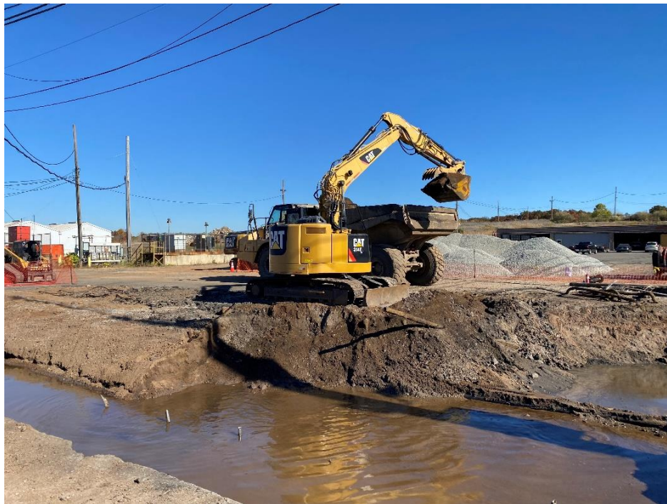
Photo 2: View of excavated soil transport to staging area in Excavation 1, IRM 1 Western Area, facing north.
