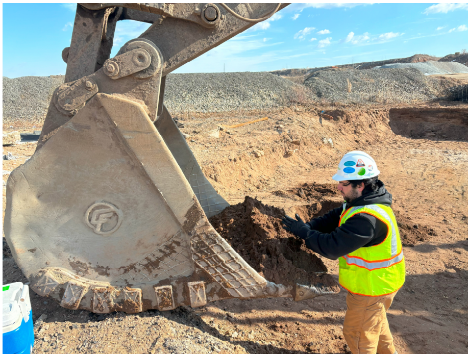
Photo 2: View of sampling activities at Excavation 12B, IRM 1 Central Area, facing northeast.
