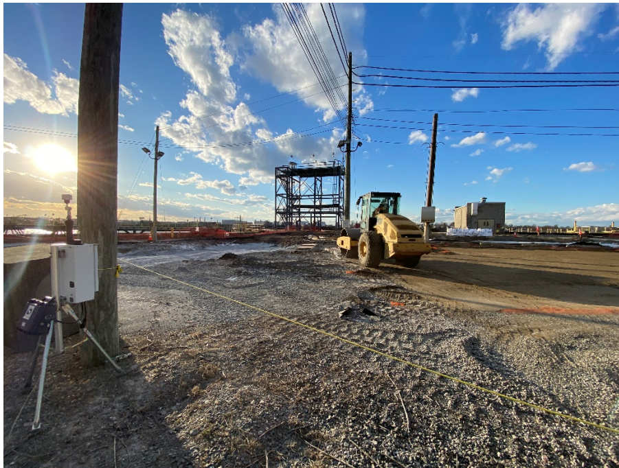
Photo 4: View of Exc. 1B backfill and compaction activities, IRM 1 Western Area, facing west.
