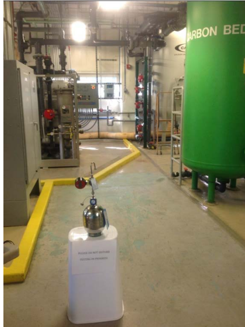
Photo #1: Sample IA1001, located in the DI Water Treatment Room.
