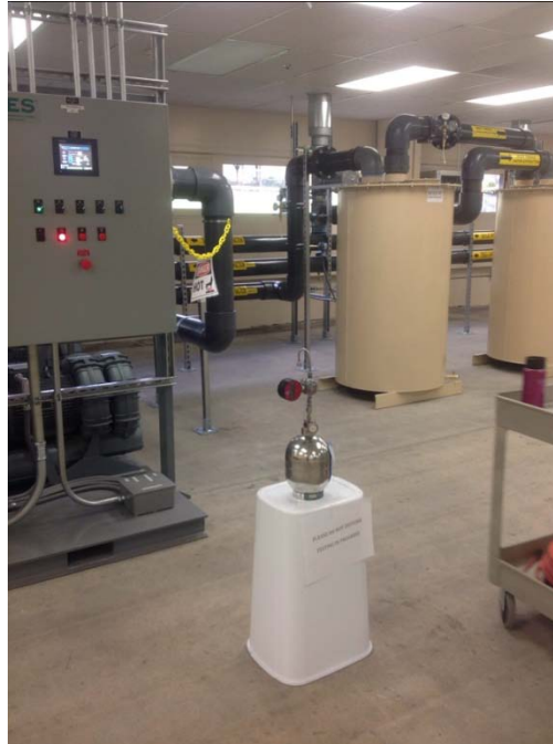
Photo #9: Sample IA1064, located in former Mail Services (subslab vapor extraction equipment room).
