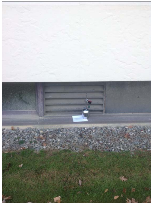
Photo #11: Sample AA1001, located at exterior intake for AHU 3-1-5.
