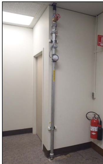
Exhibit 2: Subslab Vapor Extraction Port
