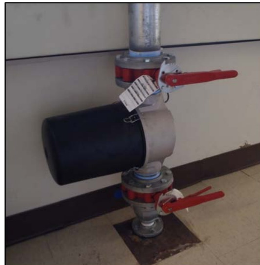
Exhibit 3: Trench Extraction Port
