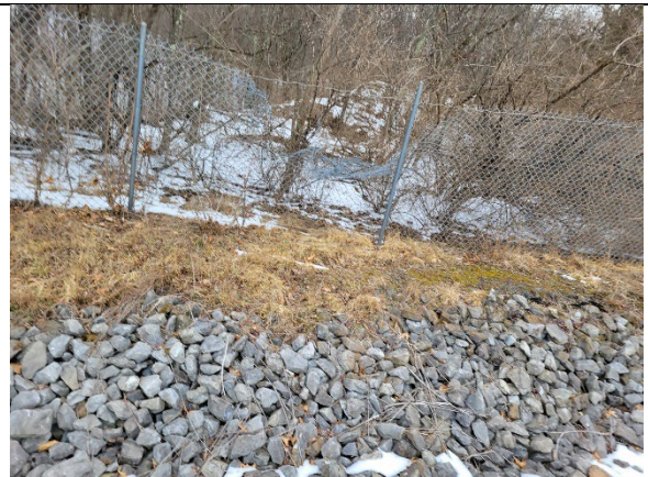
Photo 6 – Looking north at damage to the fence along the northern boundary of the landfill.
