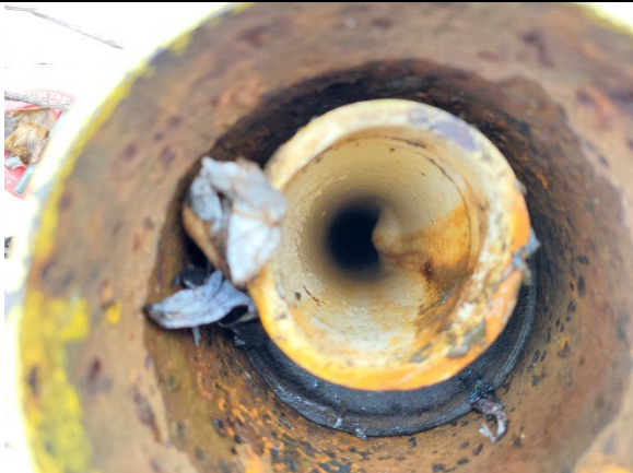
Photo 8 – Well casing damage observed in S-7.
