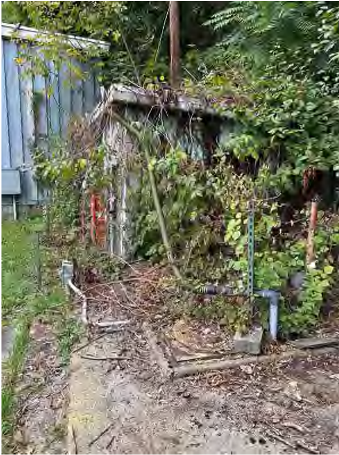
Photo Caption | Septic tank outlet left side. No pump on right side
