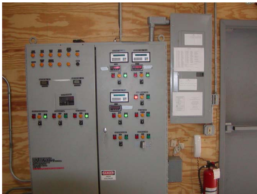
Treatment facility control panel
