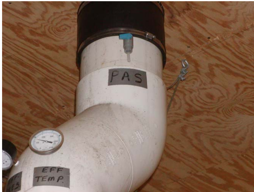
Sampling port off stack of air stripper
