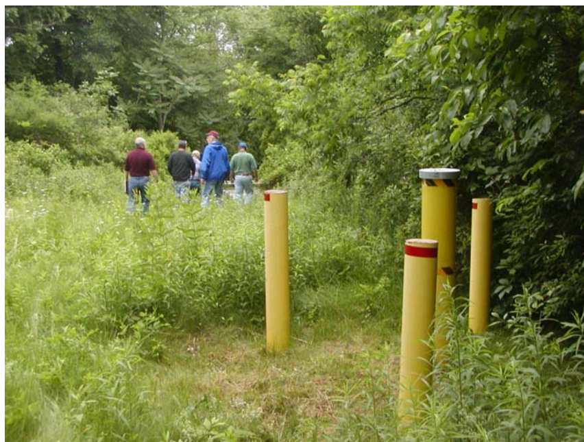
Infiltration well IW-2 (toward NYS Route 9G)
