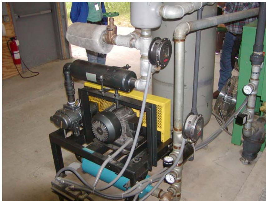
SVE vacuum skid
