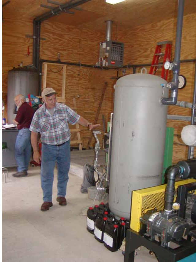
Drop-out tank and SVE vacuum/blower
