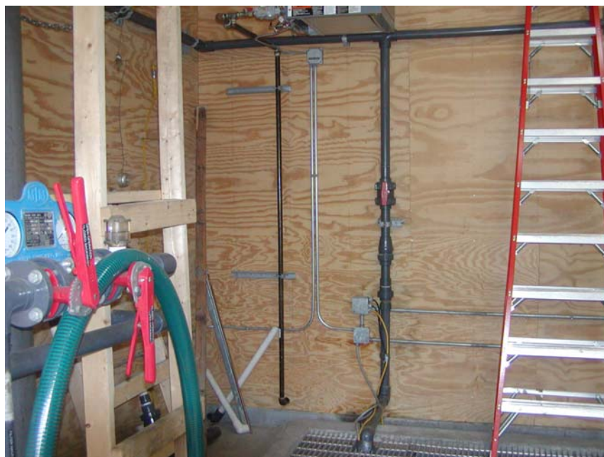
Effluent from 3 rd tank
