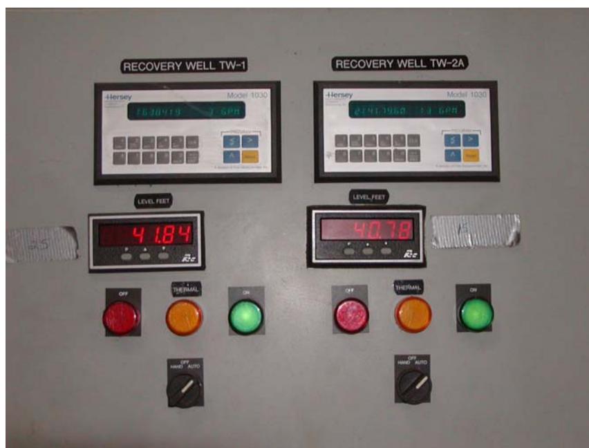
Control panel close-up; TW-1 and TW-2A totalizer, flow, and water level
