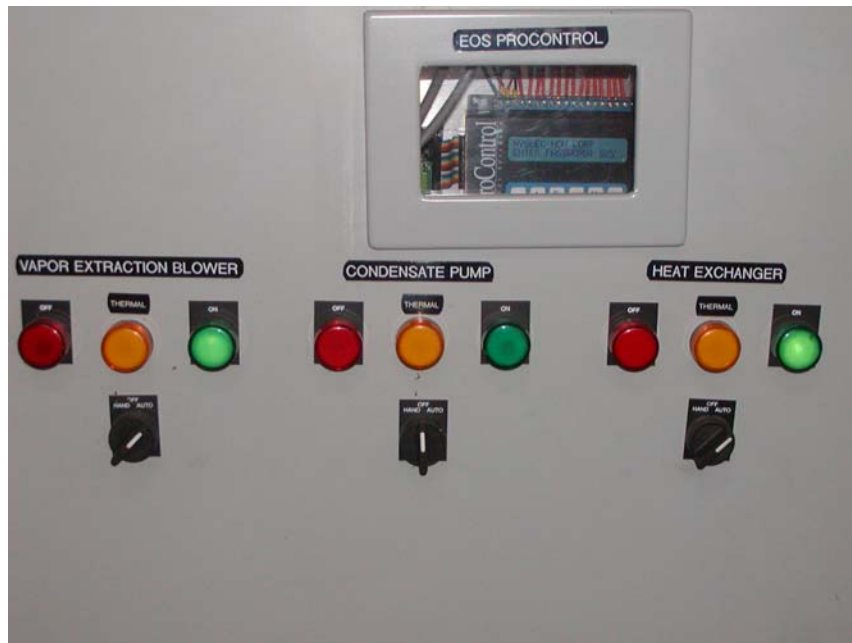
Control panel (bottom left side); vapor extraction blower condensate pump, heat exchange run lights and switches
