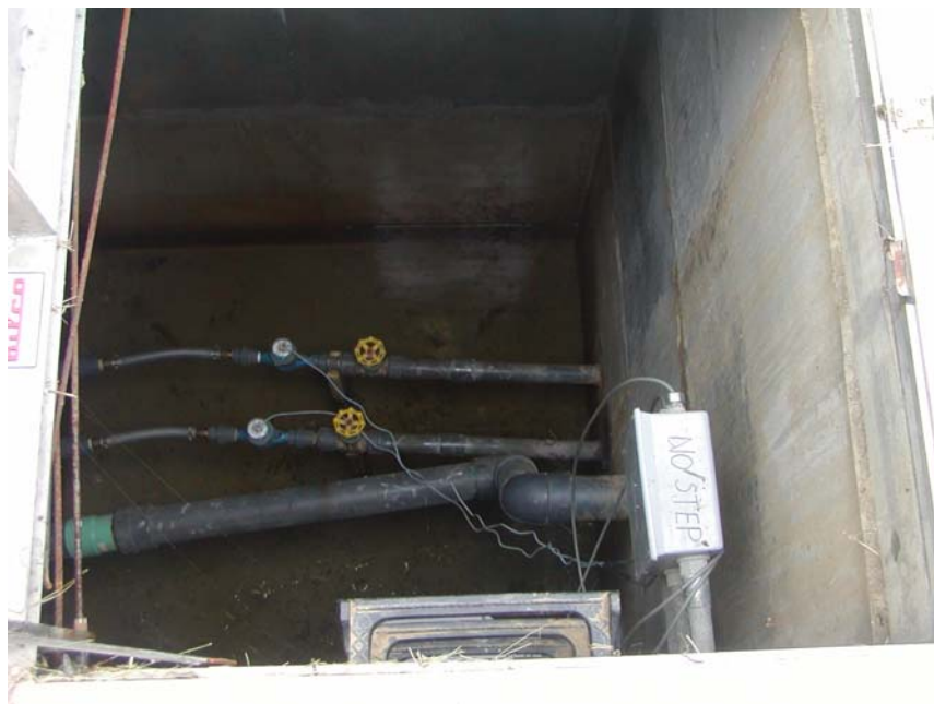
Looking down inside meter pit (effluent lines to injection wells and to the creek)
