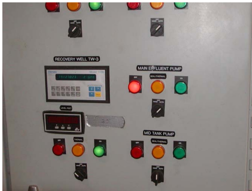
Control panel close-up; TW-3 totalizer, flow and water level (transducer is down and needs repair during this visit); main effluent pump
