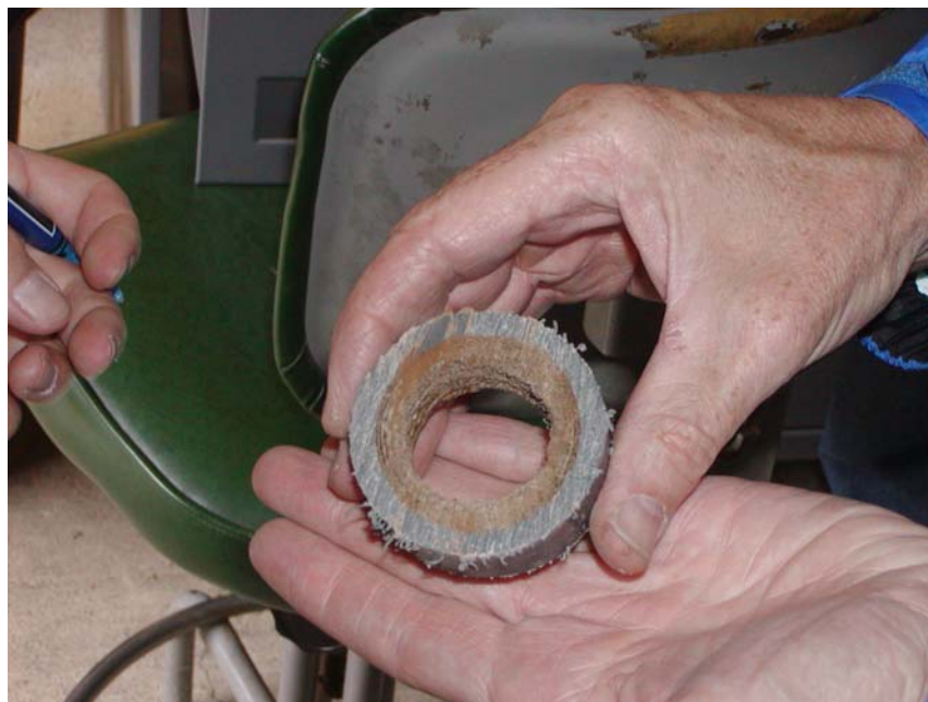
Scale build-up in piping off sandfilter
