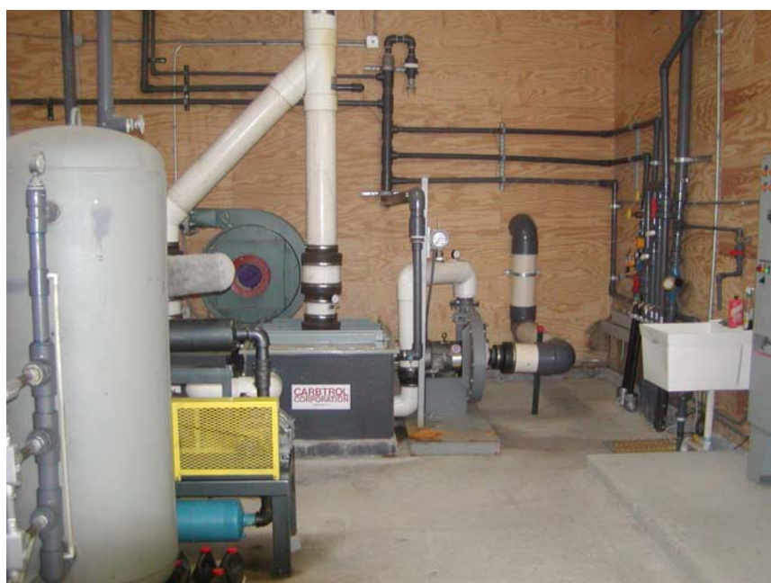
Air stripper, influent lines
