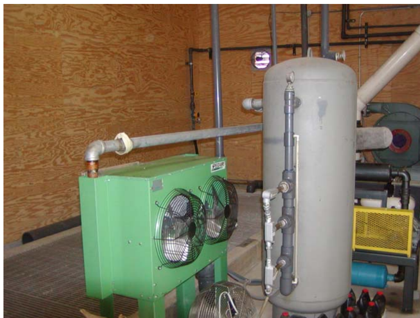
Heat exchanger and dropout tank
