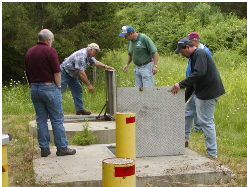
Distribution and meter pits and infiltration well, looking SE.
