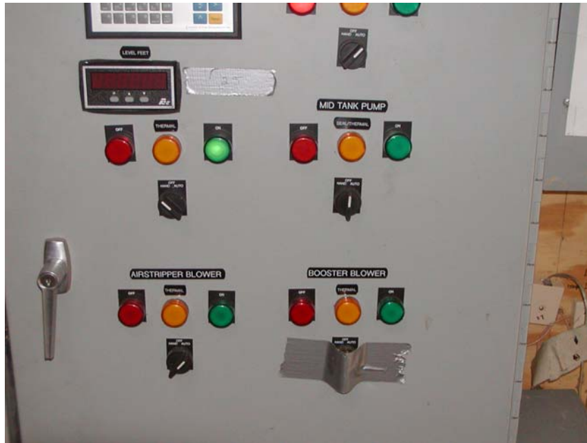
Control panel close-up; air stripper blower, booster blower (not needed any more)
