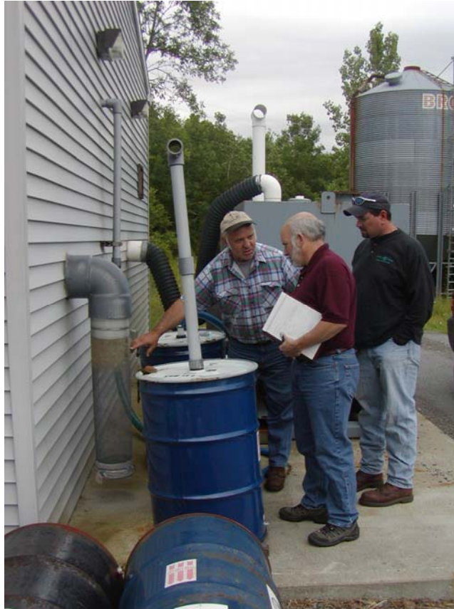
SVE GAC drums and stripper air intake
