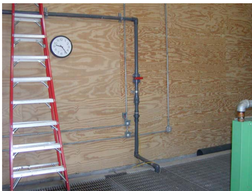
Bypass line from middle tank
