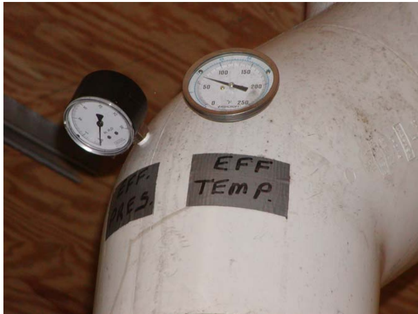
Stack temperature and pressure gages on stack from stripper
