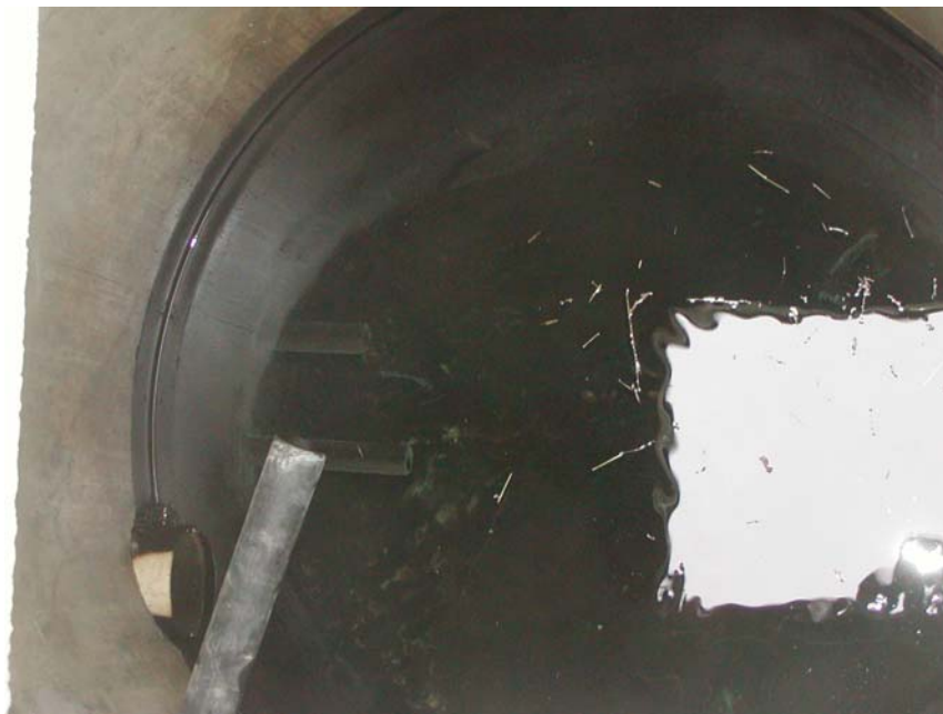
Looking down inside effluent clearwell/ distribution box. Influent lines from treatment facility (longer pipe above water), two effluent lines to infiltration wells (submerged), effluent line to creek (lower left corner shorter stub).
