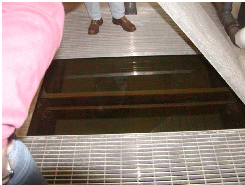
Baffle in Sediment Tank 1
