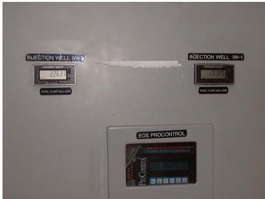
Control panel (top left side); injection well total flows for IW-2 and IW-1; window for PLC
