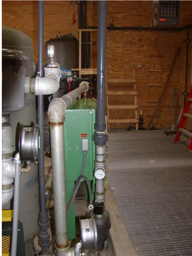
Heat exchanger (side view)
