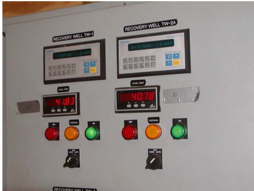
Control panel close-up; TW-1 and TW-2A totalizer, flow, and water level, different angle
