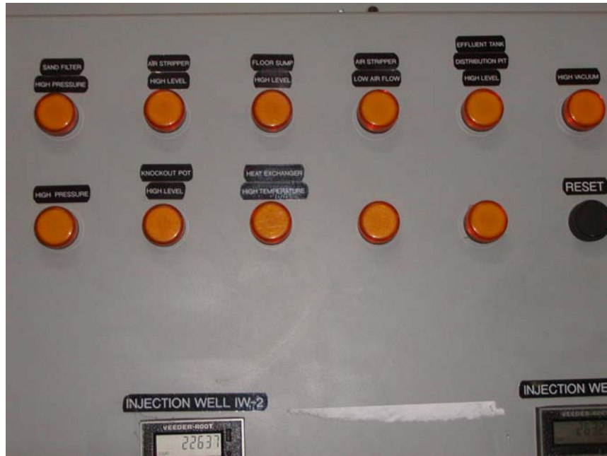
Control panel (top left side) trouble lights (different view)
