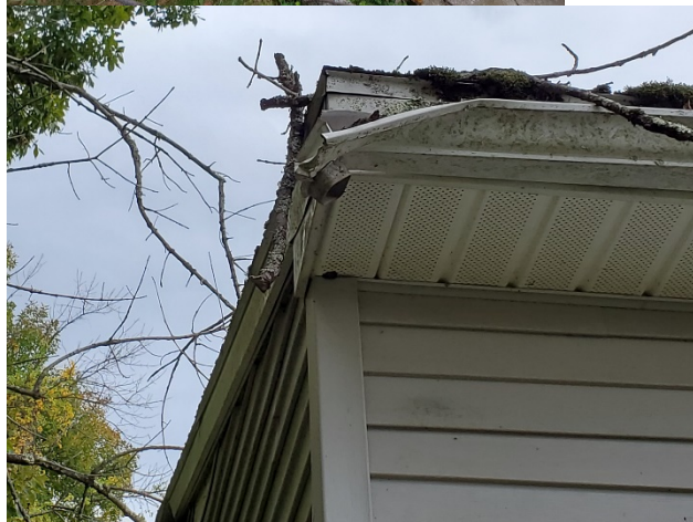
Damage to building from Limb
