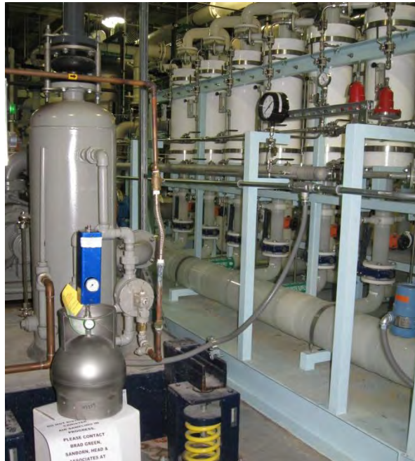
PHOTO #4 – Sample IA-0803; located in Ultra Pure Water (UPW) equipment room. Filtration tanks in background.
