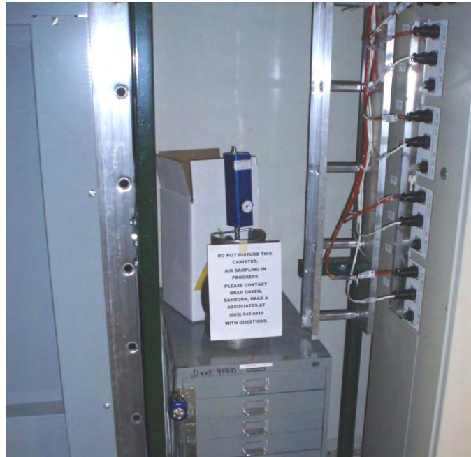
PHOTO #14 - Sample IA-0813; located in the sub-fab area near an air emission control exhaust gas scrubber.
