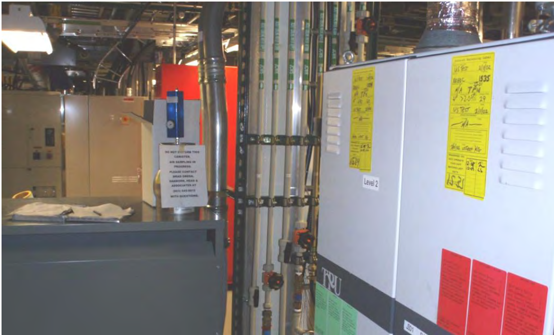
PHOTO #13 - Sample IA-0812; located in the sub-fab area near a transformer.
