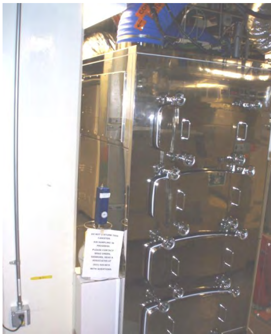
PHOTO #11 – Sample IA-0810; located in the sub-fab area near an air return unit.
