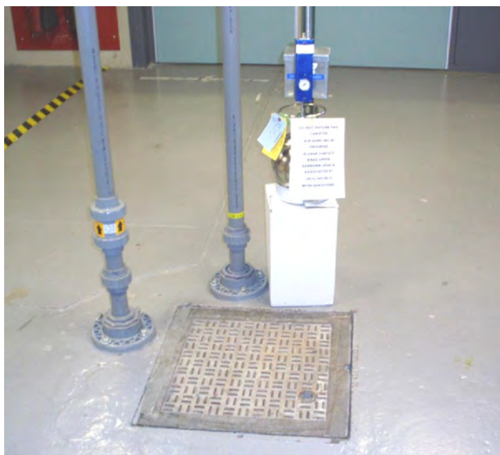
PHOTO #10 – Sample IA-0809; located in the southern part of the sub-fab area near an unused groundwater sump.
