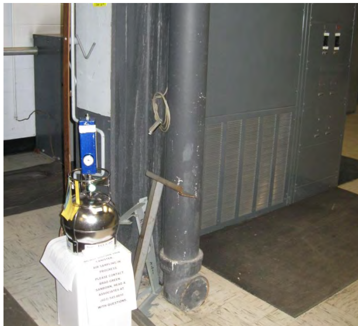
PHOTO #5 – Sample IA-1004; located in a mechanical room.
