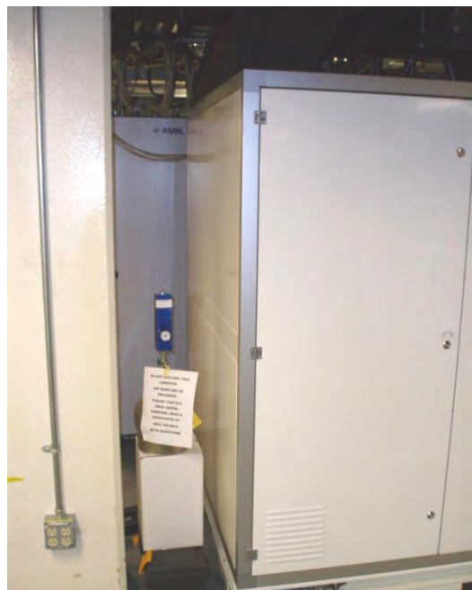
PHOTO #12 – Sample IA-0811; located in the sub-fab area near an air control unit.
