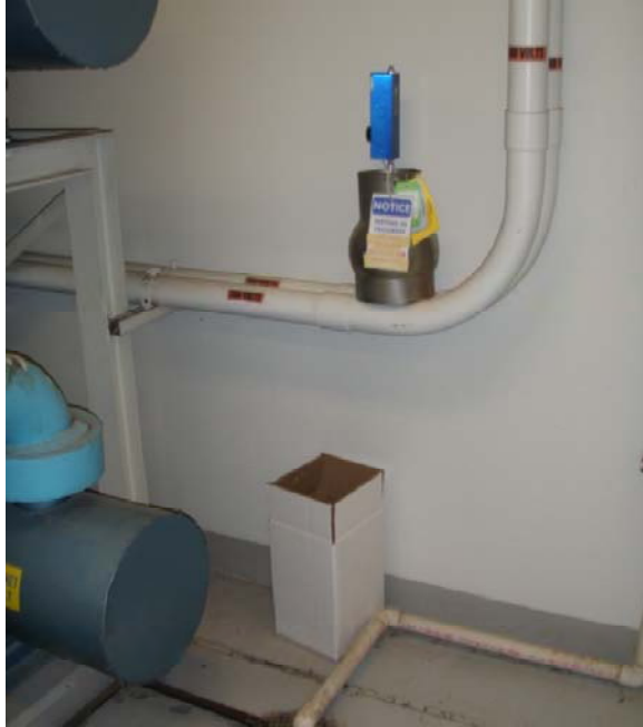
PHOTO #8 – Sample IA-0422; located in sintering manufacturing furnace room #2 near a floor discharge drain.
