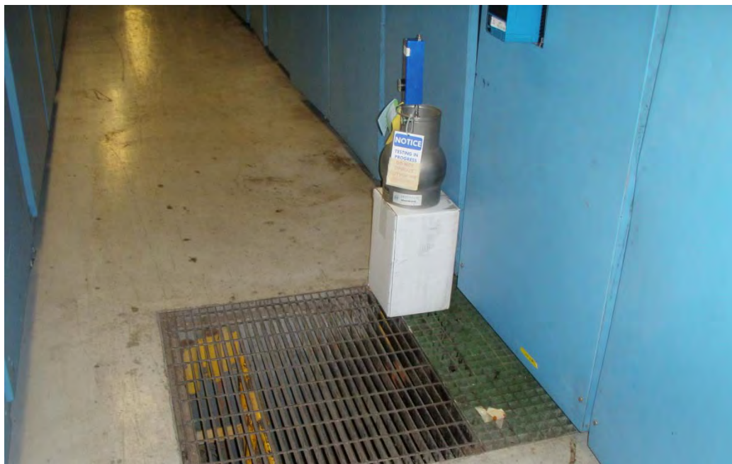
PHOTO #9 – Sample IA-0424; located in sintering manufacturing furnace room #2 near a sump.
