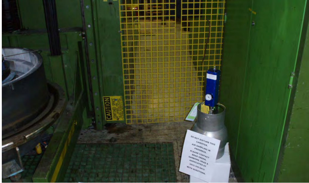
PHOTO #7 – Sample IA-0421; located in the sintering manufacturing furnace room #2 near a sump.
