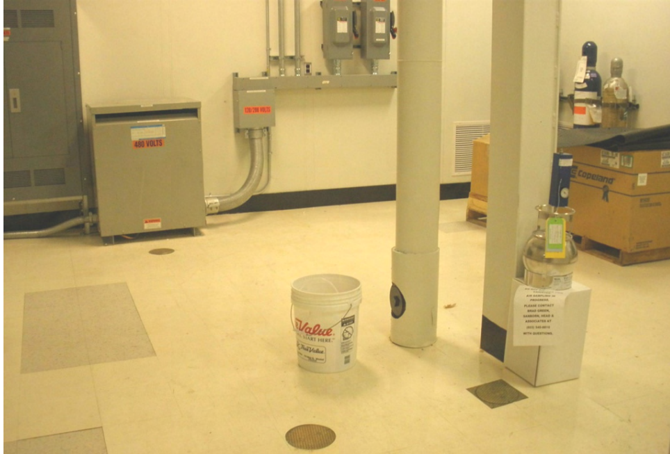
PHOTO #3 – Sample IA-0402; located in a server/storage room.
