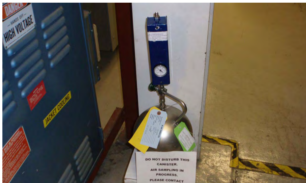
PHOTO #5 – Sample IA-0414; located in the sintering manufacturing furnace room #1.
