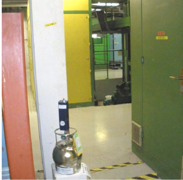
PHOTO #15 – Sample IA-0414; located in the Sintering Manufacturing Furnace Room #1.
