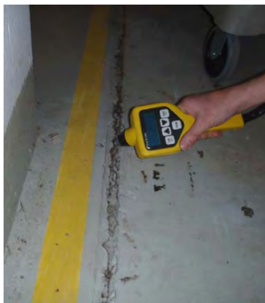
View of portable GC/MS indoor air screening at location IA0416 (left), and example of targeted air screening of an expansion joint at location TA-106 (right).
