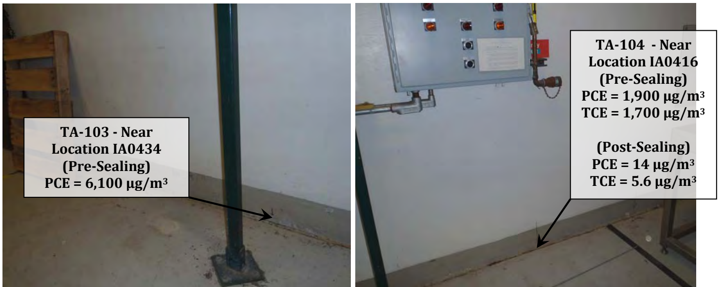
Targeted field screening results from expansion joint cracks directly below locations IA0434 (left) and IA0416 (right) under normal HVAC conditions.
