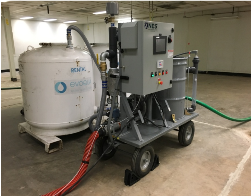
Exhibit 1 – Temporary SSDS Setup in Baseline Area of B330C
