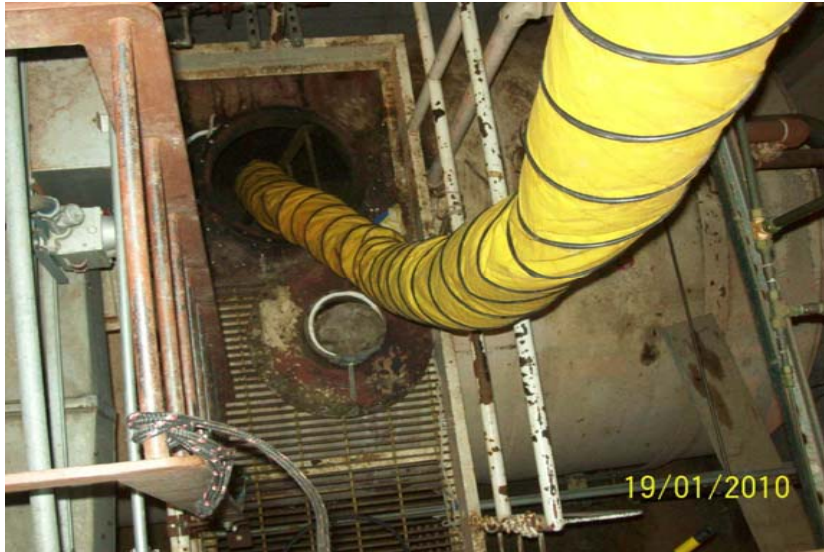
Tank 204 with the air blower to force in fresh air.
