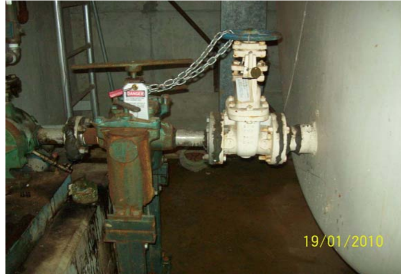
Tank 204 discharge piping was LOTO.
