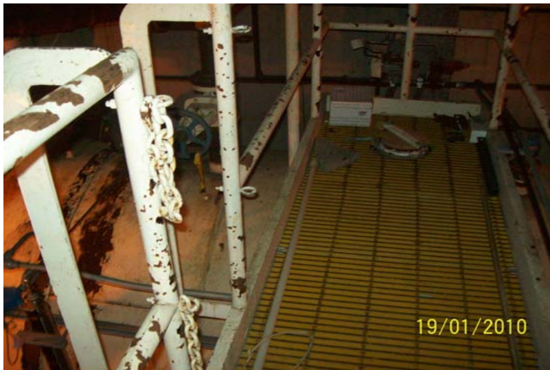
A view of Tank 207 from the catwalk.
