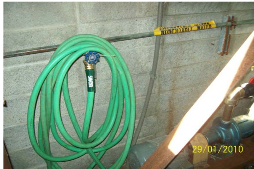
The water source from the non-potable water line of B/312 used to decontaminate the SWMUs.
