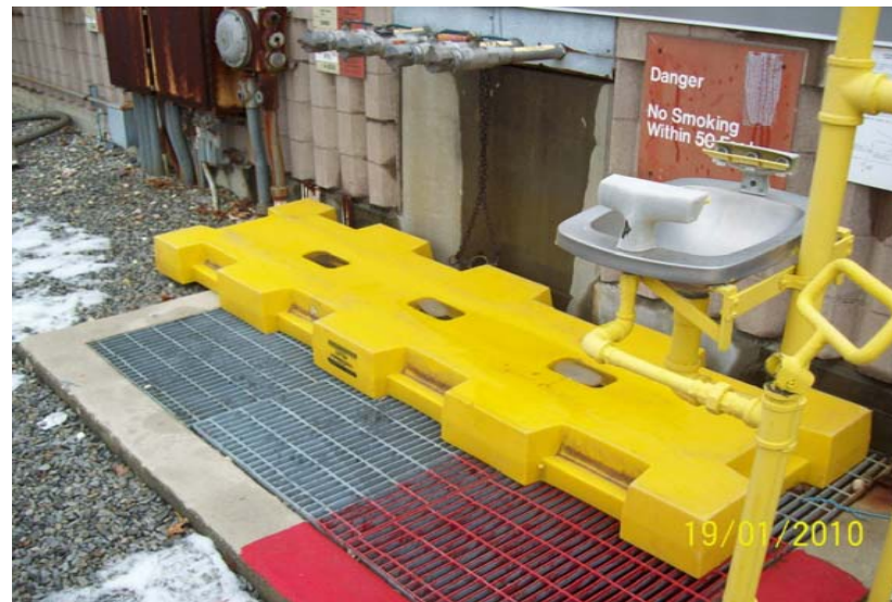
B/312B transfer area
