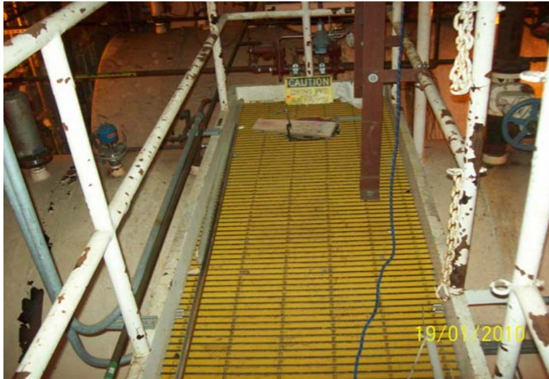
A view of Tank 206 from the catwalk.
