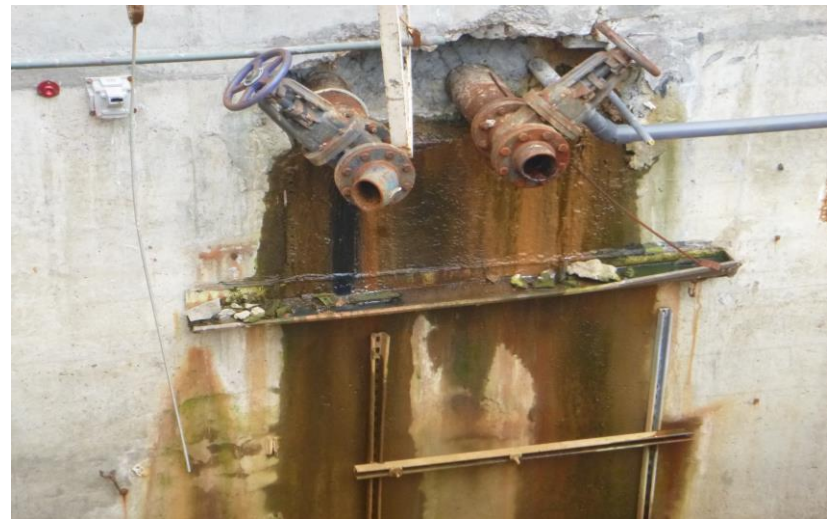
A view of the water infiltration from below the pipes along the west wall of the Solvent Vault.
