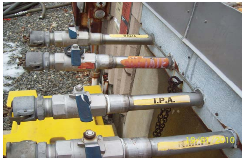
B/312B discharge piping located at the transfer area.
