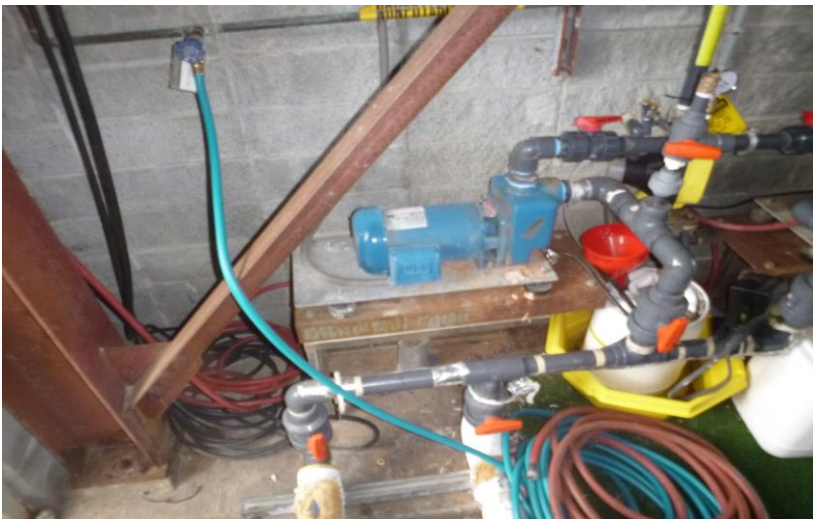
The water source from the non-potable water line in B/312 used to decontaminate the Solvent Vault and for the rinse water samples.
