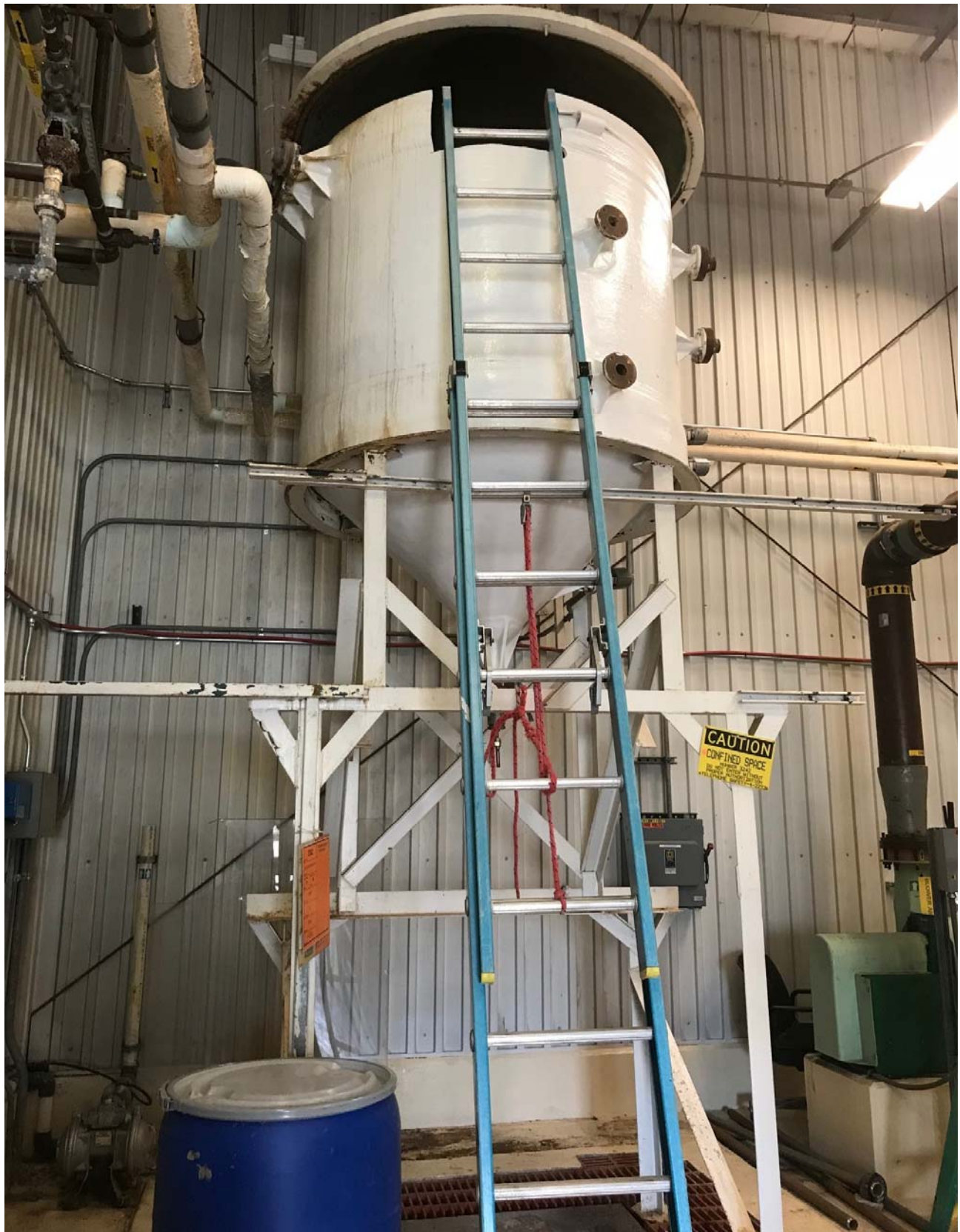
Photograph 2: SWMU 3242, solvent separator tank at the time of sampling on April 27, 2018.
