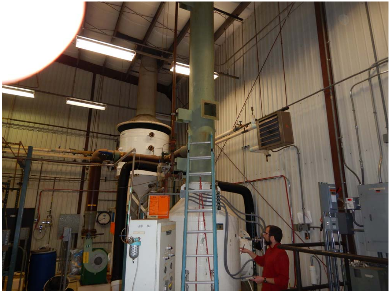
Photograph 4: SWMU 3198 air stripper effluent tank and associated air stripping tower at the time of sampling on April 27, 2018.
