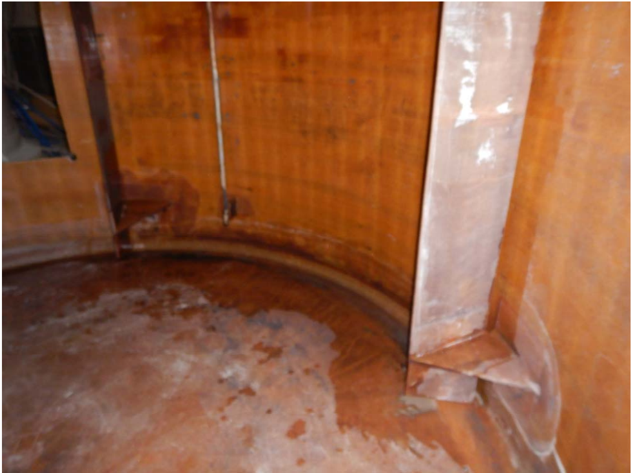
Photograph 6: SWMU 231, effluent storage tank at the time of sampling on April 27, 2018.
