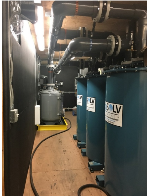
Exhibit 3.2: System VE-1 Equipment Enclosure Interior
