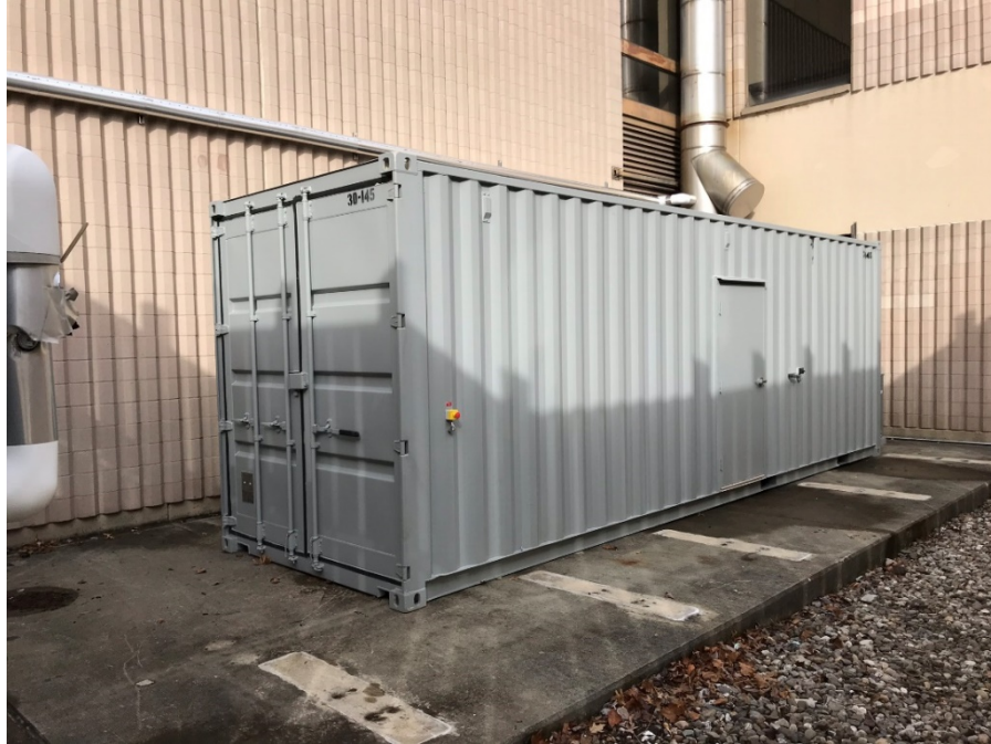
Exhibit 3.1: System VE-1 Equipment Enclosure Exterior
