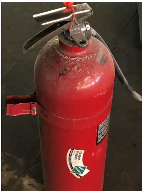
Photo #1: Carbon Dioxide Fire Extinguisher near location IA-07 in Building 310 (220)
