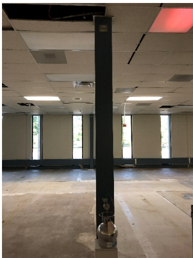
Sample Location IA-12, Column AG4 Bldg. 320A (210)
