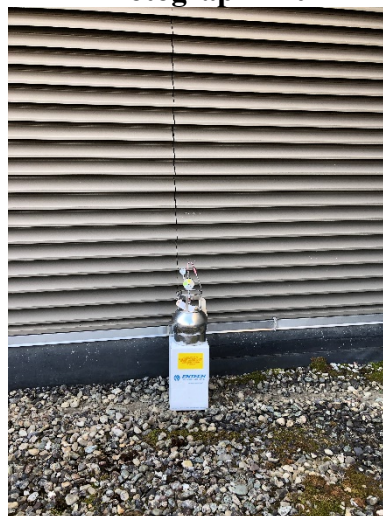
Sample Location AA-01, Rooftop HVAC Unit
