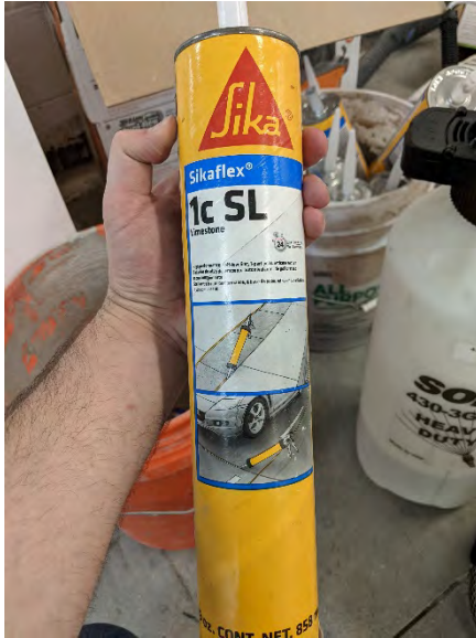
Photo #1: Sikaflex Was Being Used Throughout Open Tenant Space
