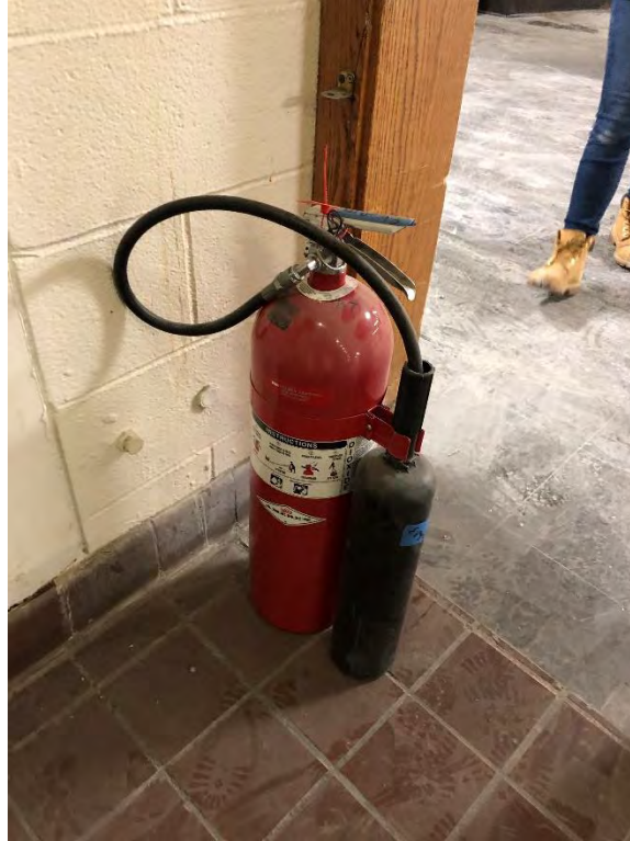
Photograph 17 CO2 Fire Extinguisher – Column T-14
