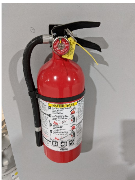
Photo #3: Type B:C Fire Extinguishers throughout Midway space
