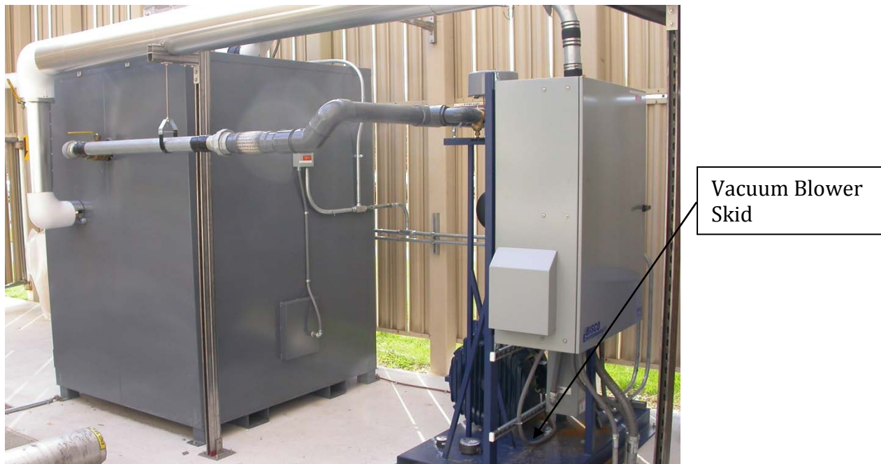
Photo 9: Blower skid and heated enclosure – located outside the 80K area of B330D
