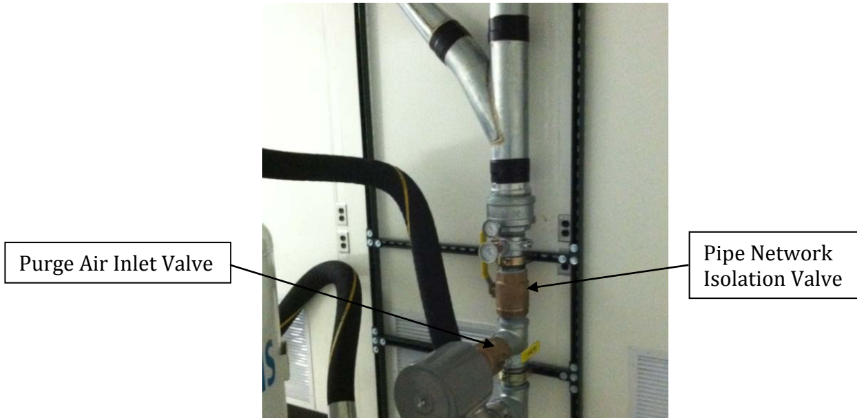
Photo 1: Piping from extraction ports to GAC vessels including pipe network isolation valve (open) and purge air inlet valve (closed).
