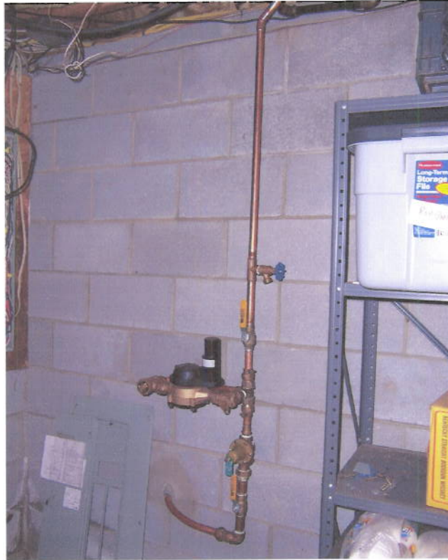
Municipal water connection in basement of Lot 9. 10-3-08.
