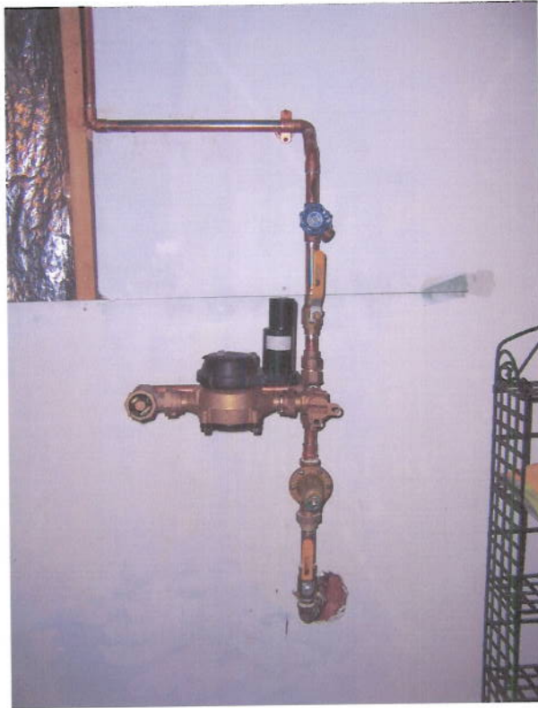
Municipal water connection in basement of Lot 10. 9-30-08.
