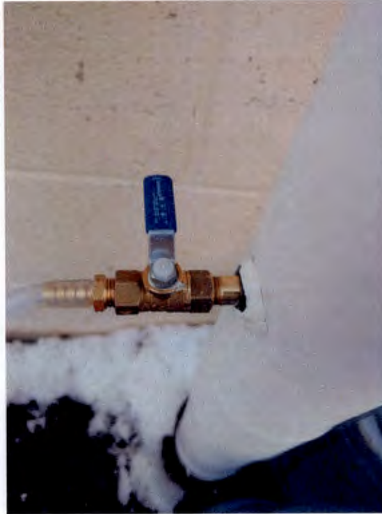
Photograph 3: Sample SSDS-W sample port with shut-off valve. Shut-off valve shown in “off” position and turned on prior to sampling.
