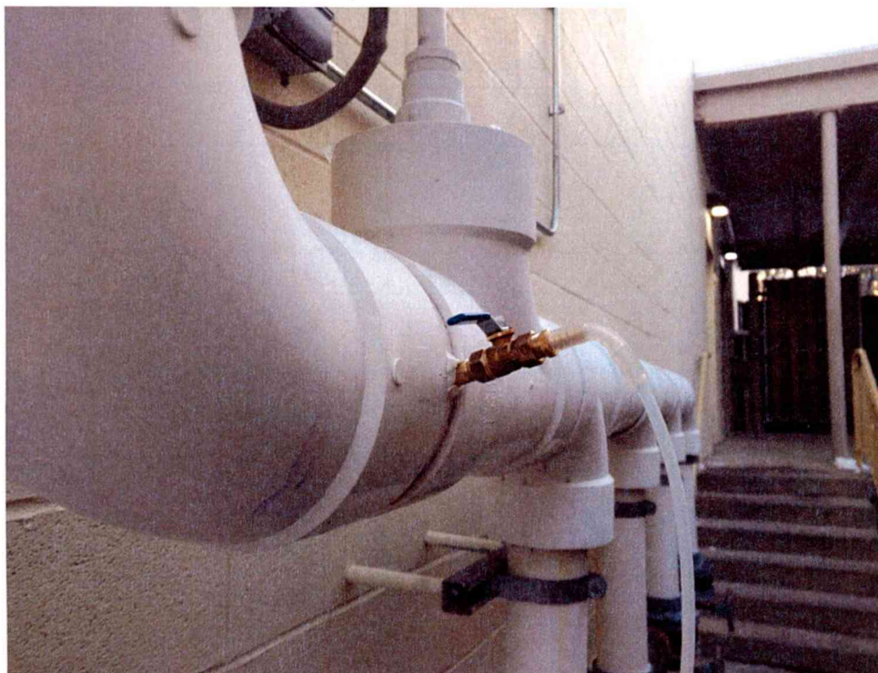
Photograph 5: Sample SSDS-E sample port with shut-off valve. Shut-off valve shown in "off" position and turned on prior to sampling.
