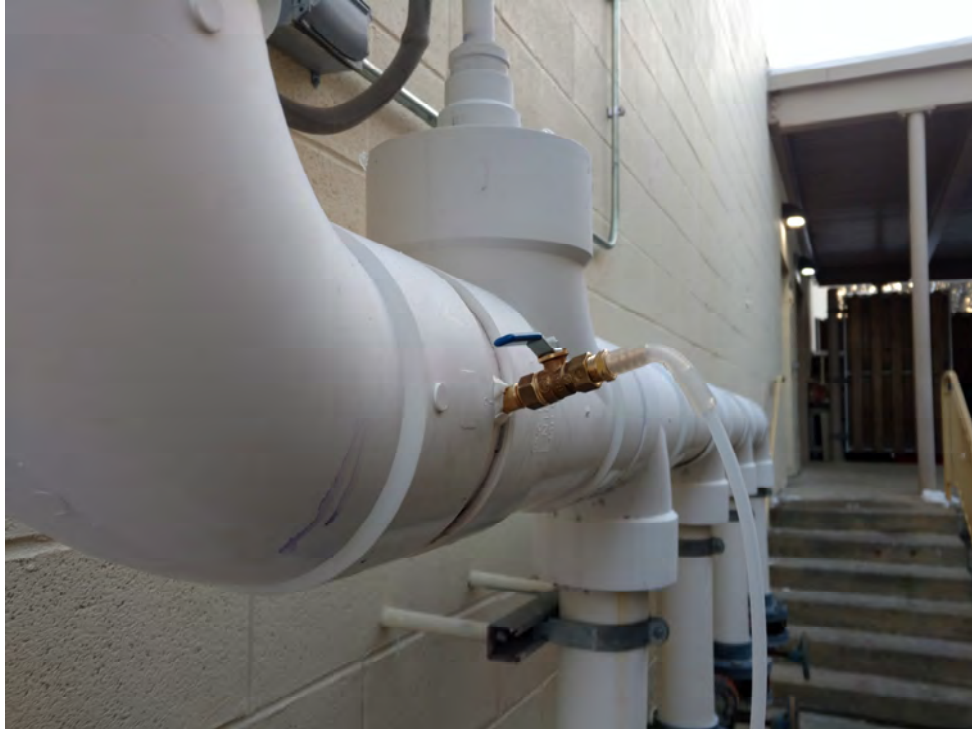
Photograph 5: Sample SSDS-E sample port with shut-off valve. Shut-off valve shown in “off” position and turned on prior to sampling.
