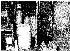
Softener & Brine Tank
