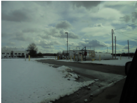
AST fuel farm, north of AAG hangar
