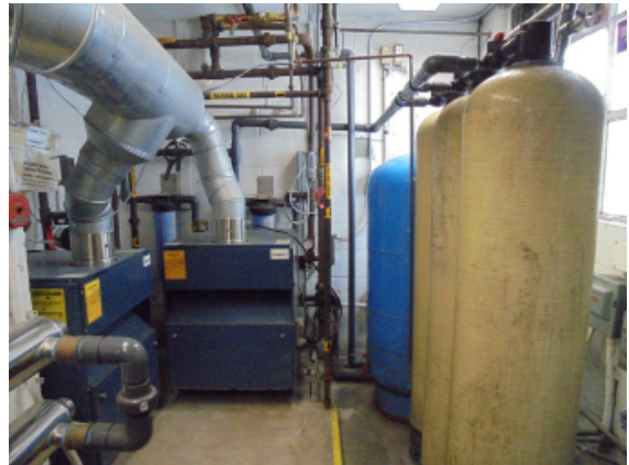
Boiler room of AAG hangar (form IBM hangar) with POET system
