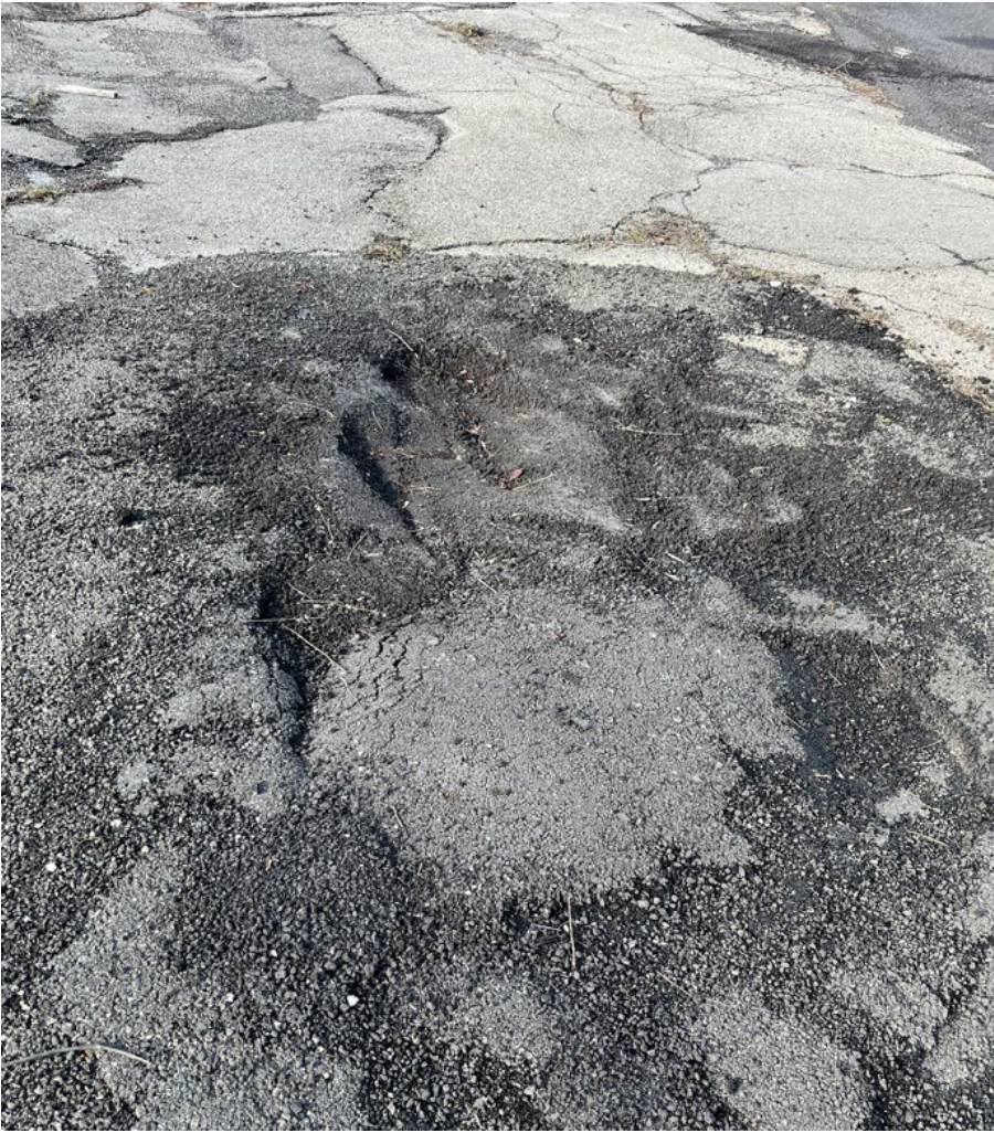
Representative patched pavement area
