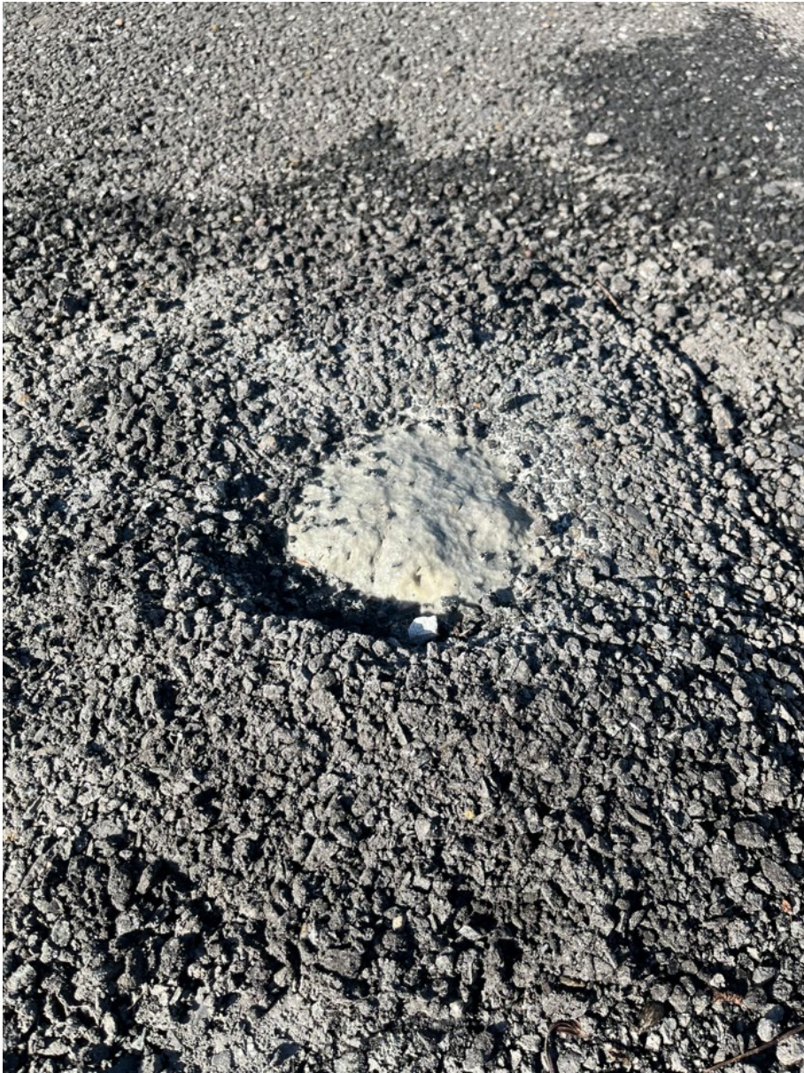
One location ~6 inches in diameter hole
