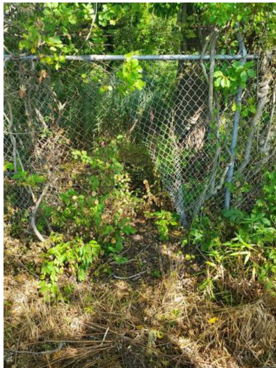
Photo 14: Fence along northern site border prior to repair of breach
