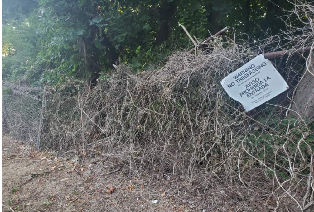
Photo 7: Fence along Pierces Road prior to repairs
