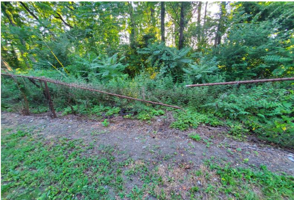
Photo 8: Fence along Pierces Road prior to repairs
