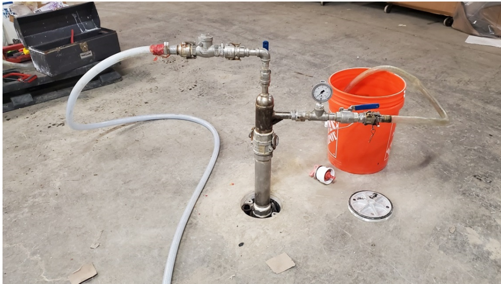
Photograph 5. ISCO wellhead connection detail.
