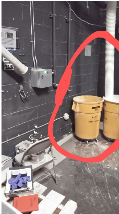
Photograph 6: Dusted area in Garbage Room (SS-SV-04/IA-04)
