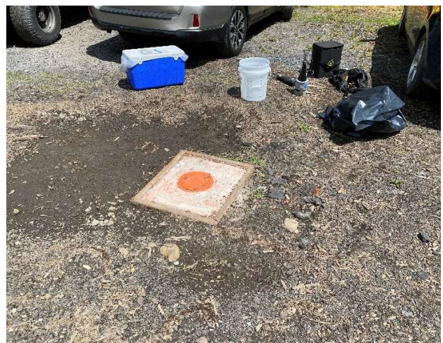
Photo 6. MW-1 replaced flush-mount.
