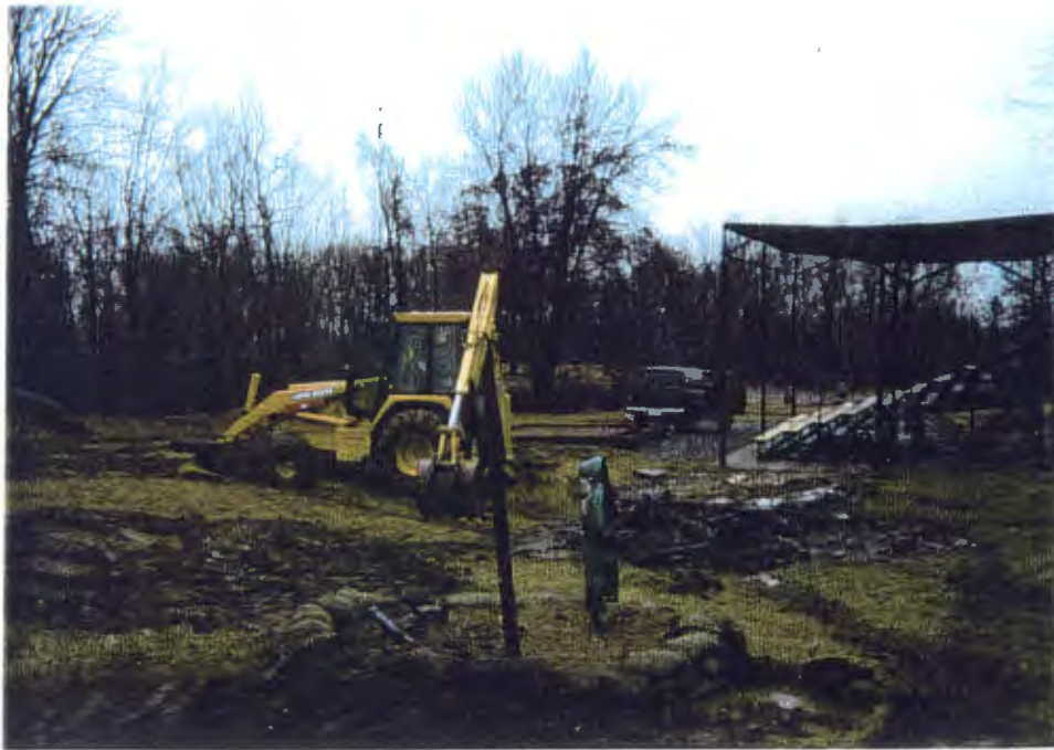
Photograph 11 Test Pit 13 - Landfill debris encountered to a depth of 12 ft. Orientation - East
