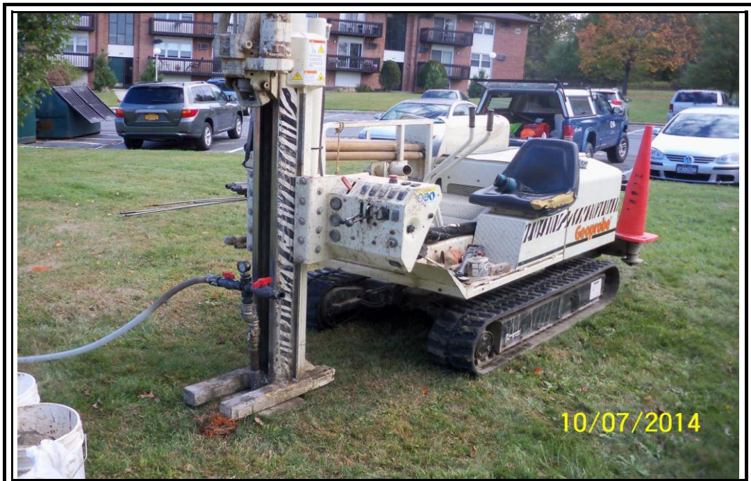
Photo 4 – View of typical 3DME injection setup, in area of monitoring well S-9
