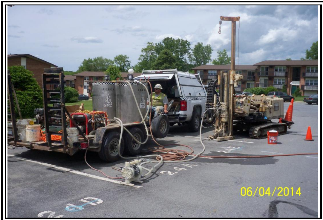
Photo 3 – View of typical PersulfOx™ injection setup, in area of monitoring well S-2
