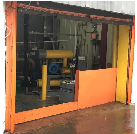
“Campbell Dams” deployed at Scrubber
