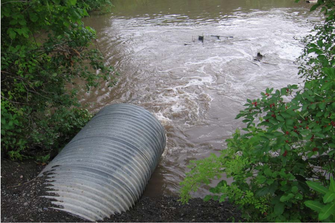
Plate 5: Culvert discharging into Little Falls Pond #2 – shows waste refuse.
