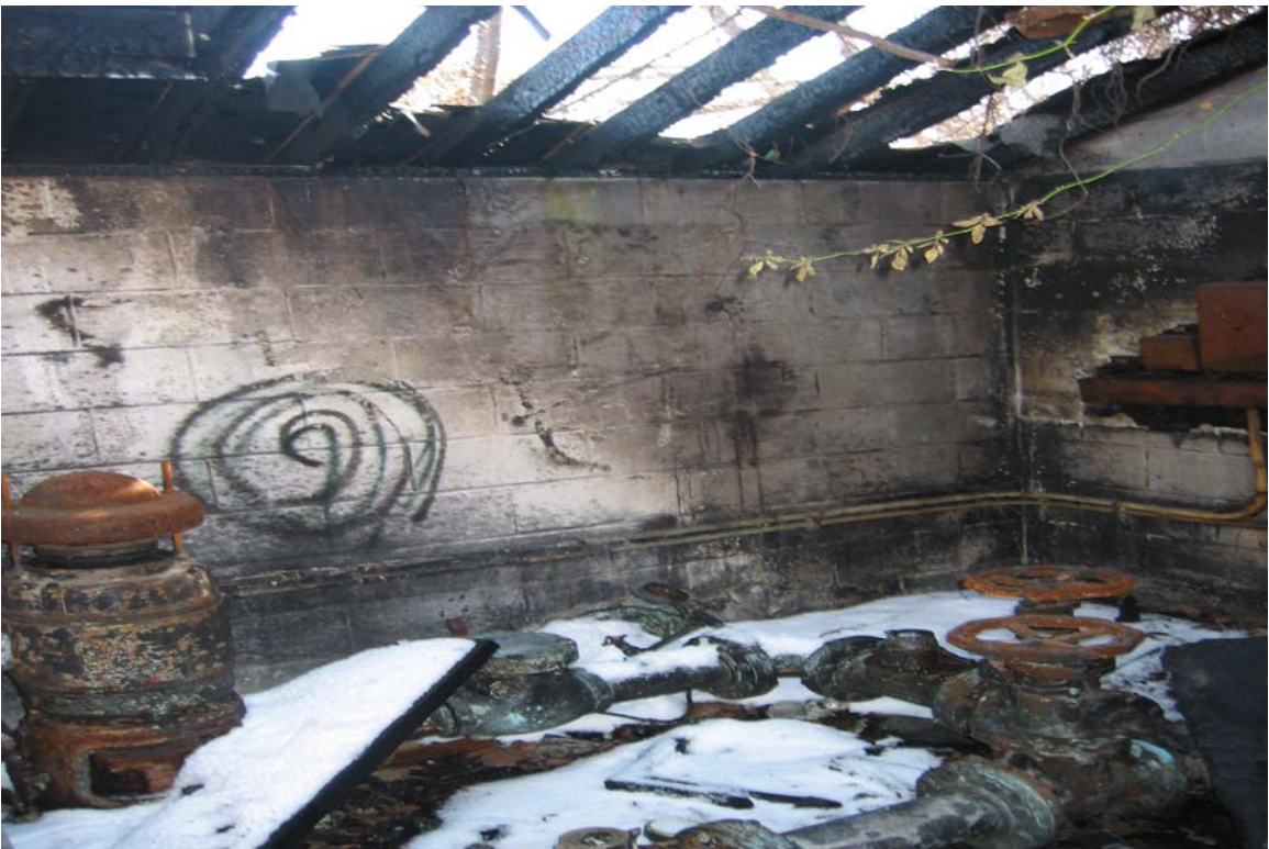
Plate 4 Condition of Former Town Pumping Well Building #1.
