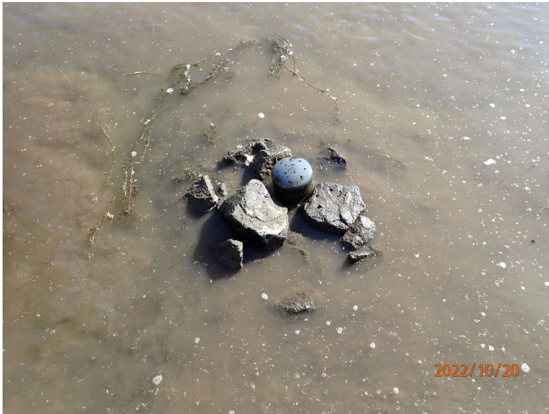
Photo 5 – Bub 4 – 4” diameter perforated pipe just above the water line with stone protection around pipe.
