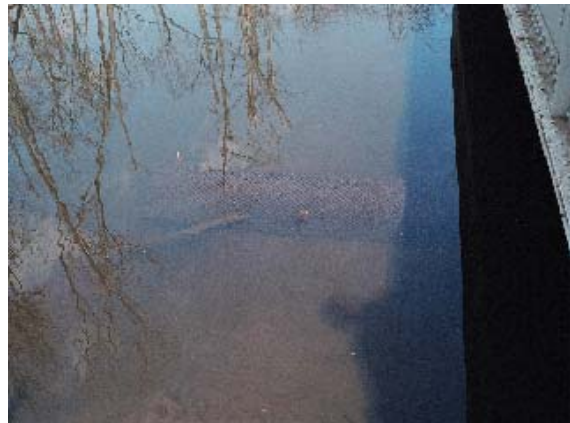
Figure 6 Drainage pipe under west side of Railroad Bridge Note that intake of pipe is covered in meshed fence material
