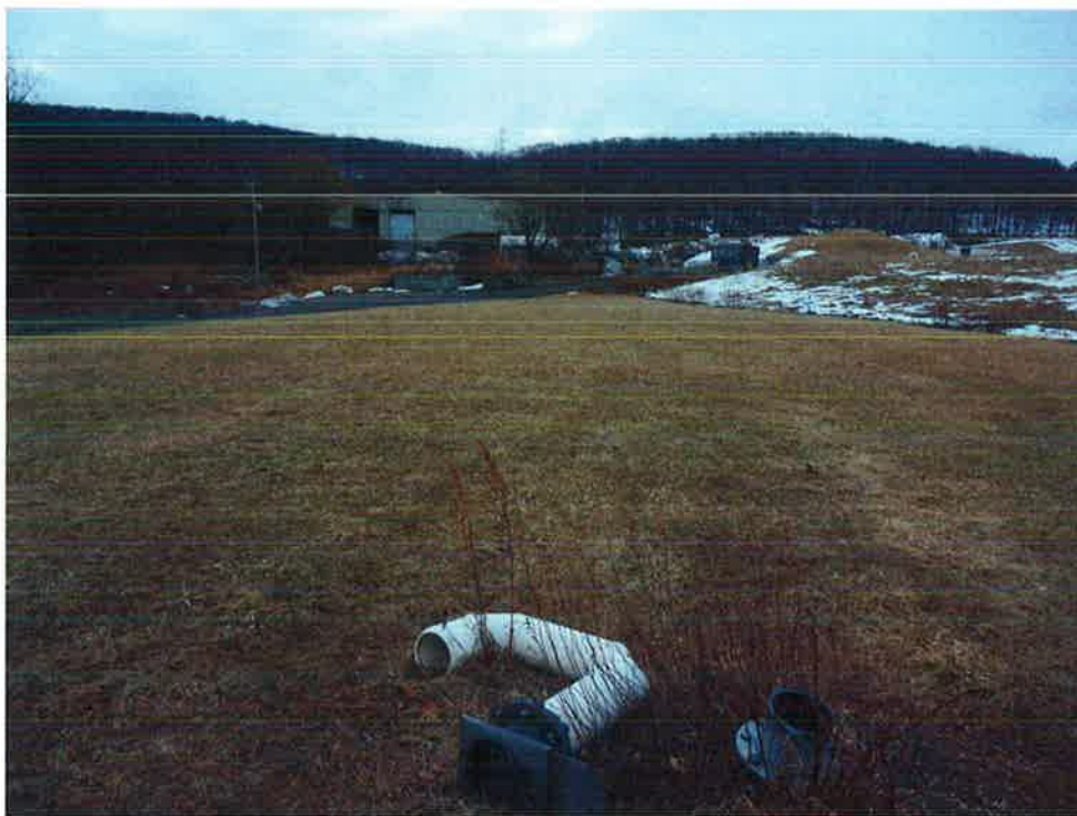
Photograph 3: Down vent on north portion of Landfill.
