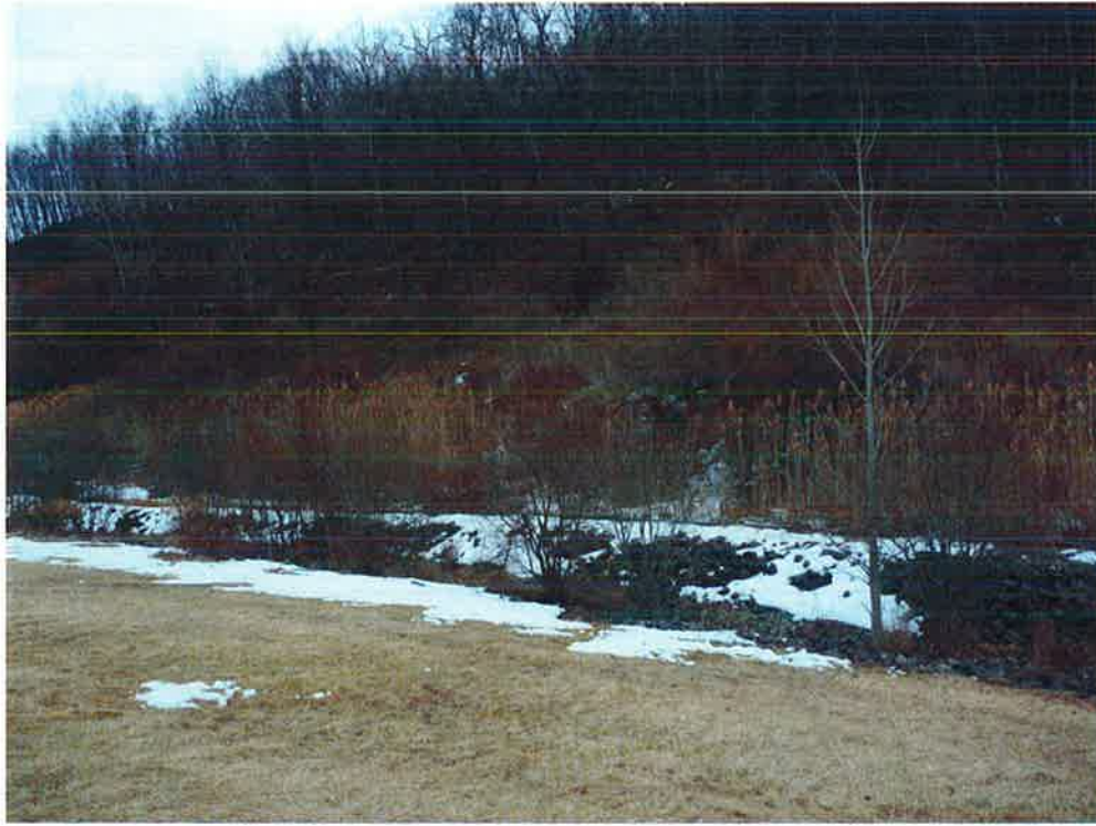
Photograph 7: Overgrown vegetation and tree present in drainage channel on southeastern border of the Landfill.
