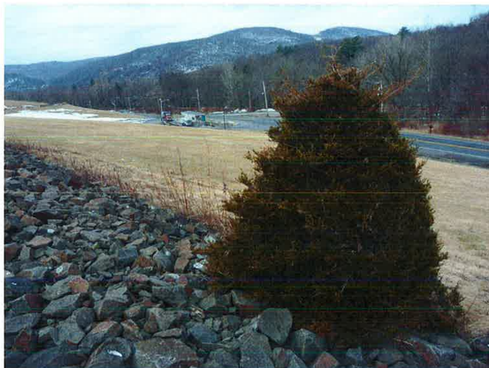
Photograph 4: Tree present in drainage swale on the northern portion of the Landfill.
