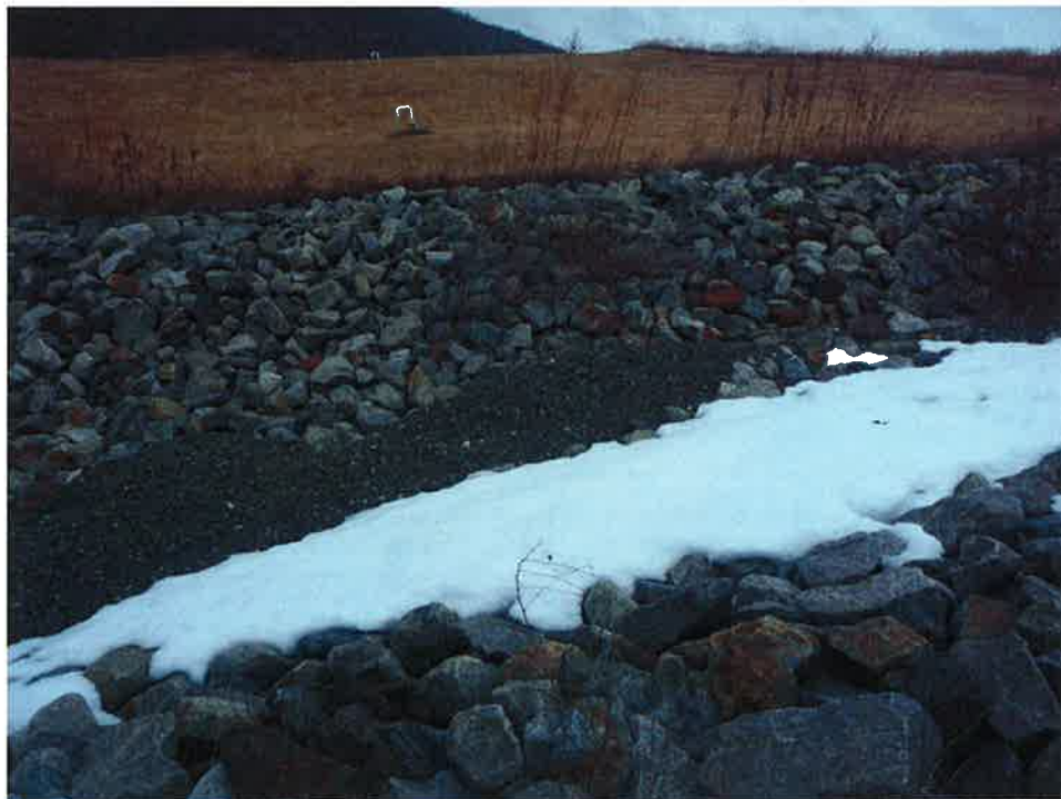
Photograph 10: Gravel is present in drainage channel from washout of Access Road on northeast portion of Landfill.
