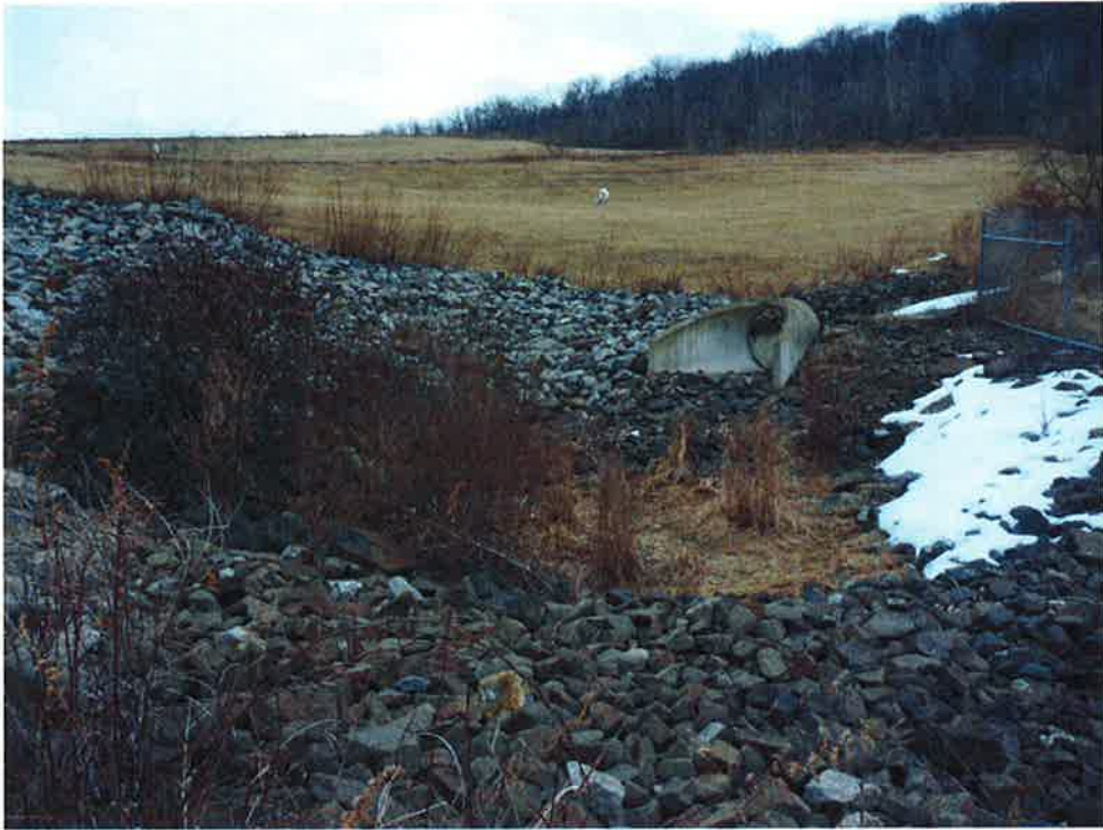
Photograph 5: Overgrown drainage channel on southwestern edge of Landfill.
