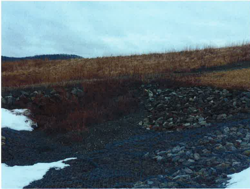
Photograph 9: View of access road in northeast portion of Landfill in background of photograph. Gravel runoff into the drainage channel.
